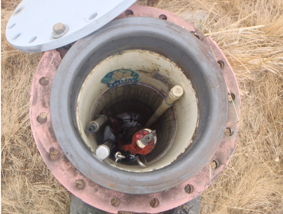
Photo 5. Condensate sump CS-5. Photograph taken on 9/21/12.
