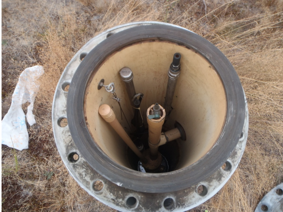
Photo 9. Condensate sump CS-9. Photograph taken on 9/21/12.
