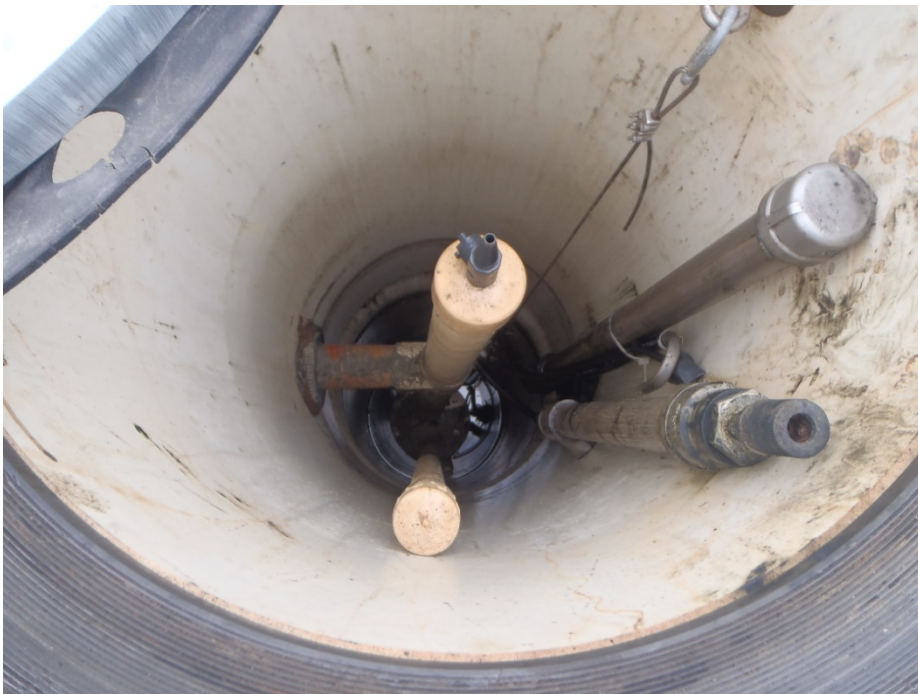
Photo 6. Condensate sump CS-6. Photograph taken on 9/21/12.
