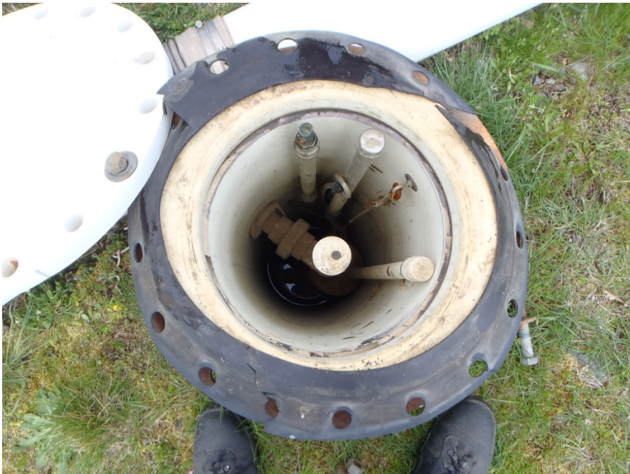
Photo 4. Condensate sump CS-4. Photograph taken on 4/27/12.
