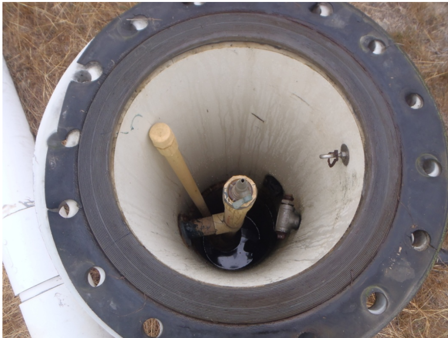
Photo 10. Condensate sump CS-10. Photograph taken on 9/21/12.
