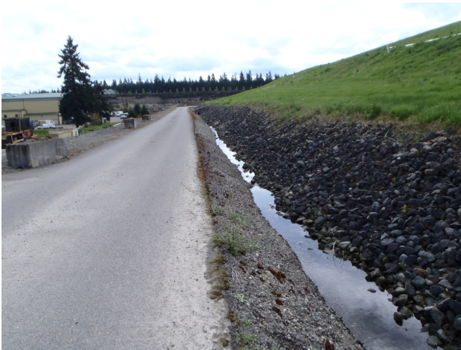
Photo 13. View of east slope of landfill, facing towards the compost facility. Photograph taken on 4/27/12.
