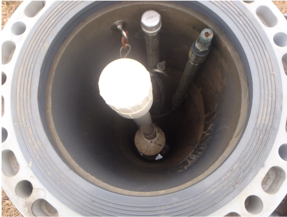
Photo 7. Condensate sump CS-7. Photograph taken on 9/21/12.
