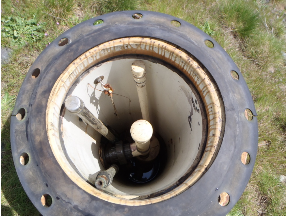
Photo 3. Condensate sump CS-3. Photograph taken on 4/27/12.
