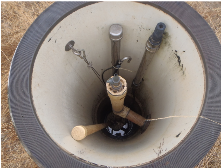
Photo 8. Condensate sump CS-8. Photograph taken on 9/21/12.
