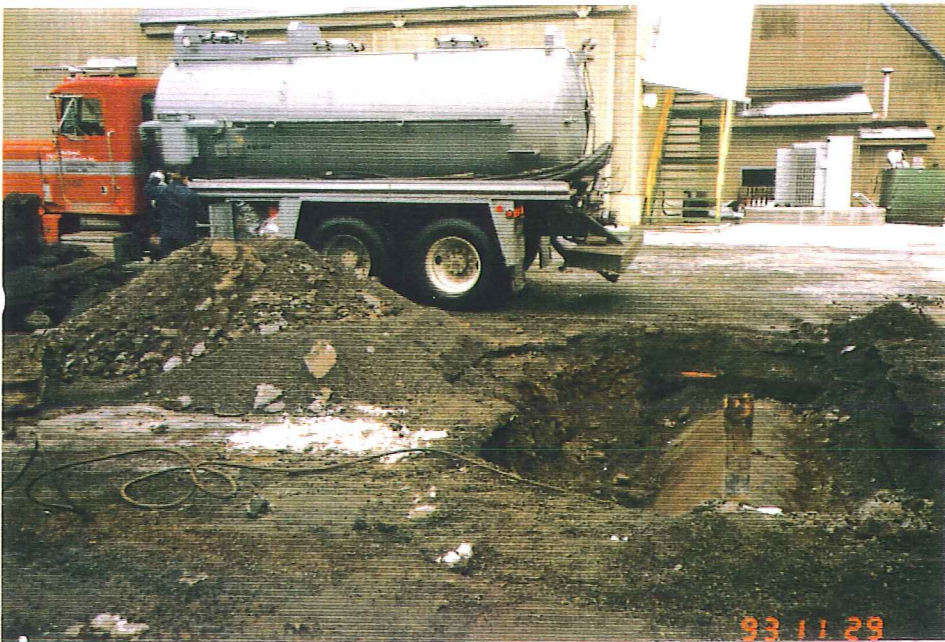
Photo 2. The tank was inerted by Sound Testing, Inc., Seattle, Washington. Line in foreground connects to purging equipment.
