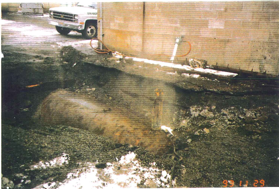
Photo 1. Site underground storage tank. Small building housing heat exchanger in background.
