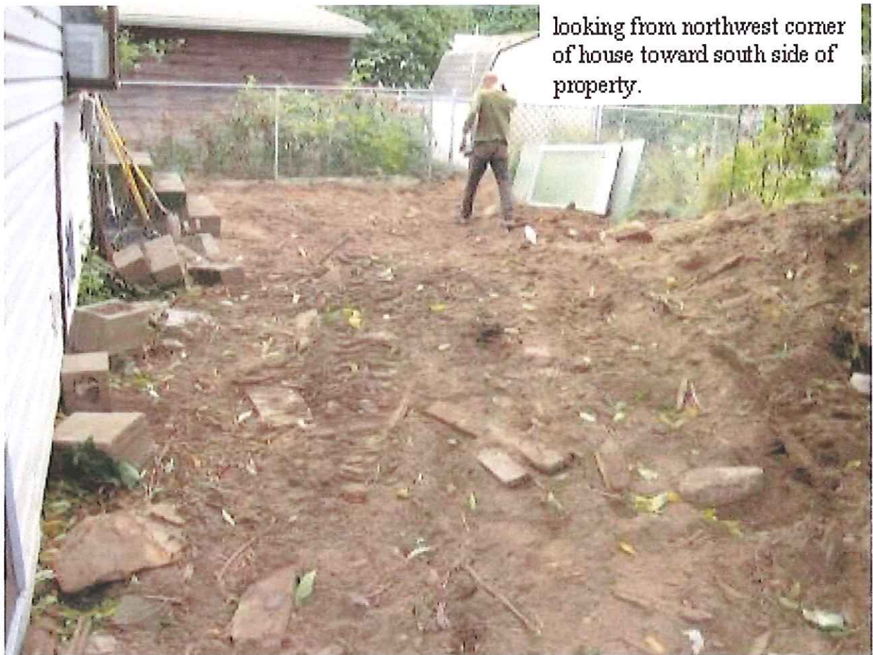
looking from house to back of flat bed trailer on site loaded with prunings from tree.
