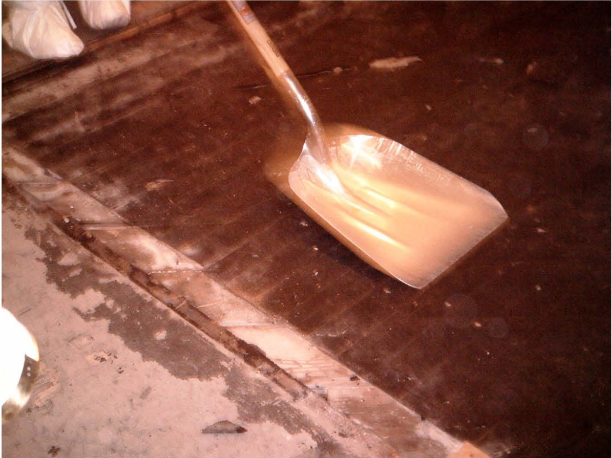
Figure 13 Previously Removed Wall Penetrating Flooring
