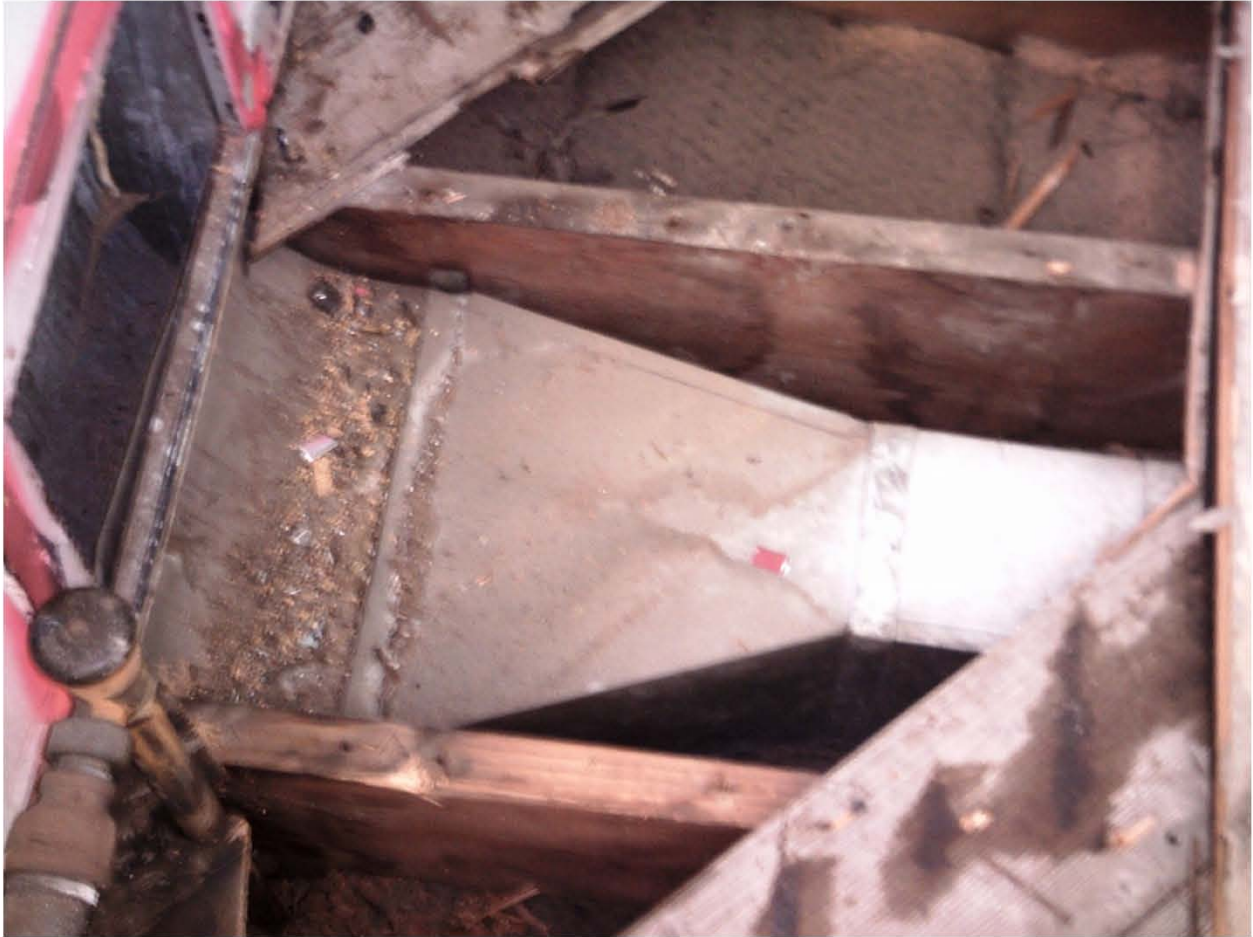
Figure 16 West Floor Exhaust Vent
