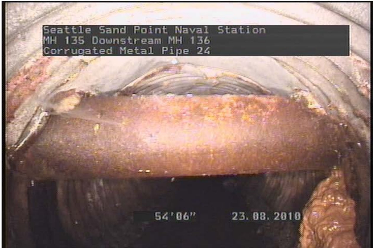
Figure 27 24 Inch Storm Sewer Line Obstruction near Catch Basin CB-1
