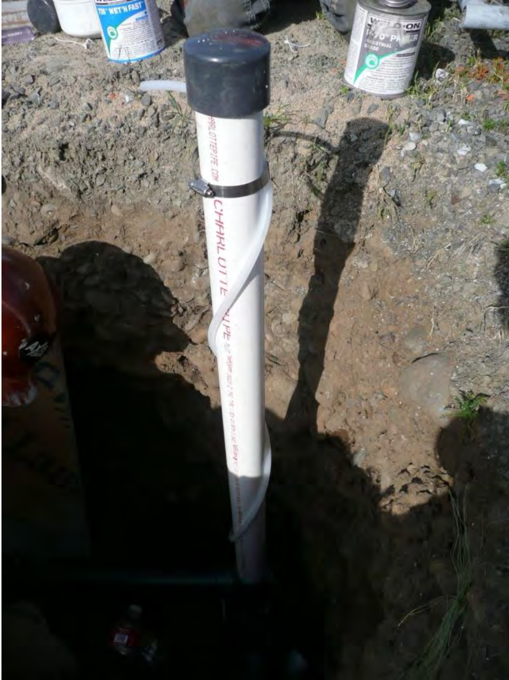
Photo 20 - Tubing to measure pressure and/or vapors from upper zone 4-inch annular space. 5/01/12
