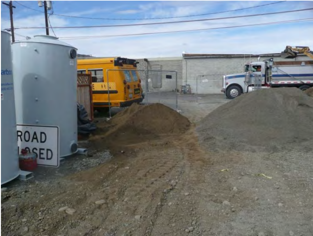
Photo 54 - GAC cans to be placed on concrete pad outside of utility building. Bedding sand and 5/8-inch crushed stone top course or structural fill. 6/08/12
