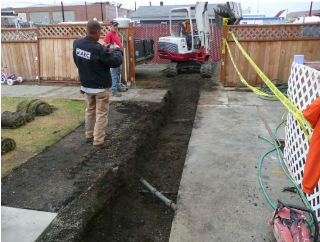
Photo 66 - Re-excavating second half of playground to remove impacted 1-1/4-inch import to clean 5/8-inch material on northern side of fence. Chemical analysis detected PAHs in previous confirmation samples. Replacing with clean 5/8-inch CSTC. 6/26/12
