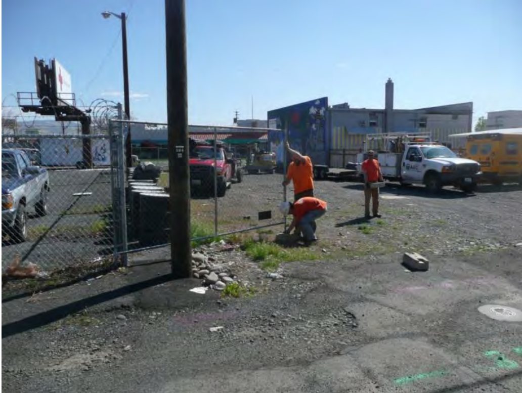
Photo 1 – Anderson Environmental Contractors (AEC) mobilizing to the site and securing with fence. 4/23/12
