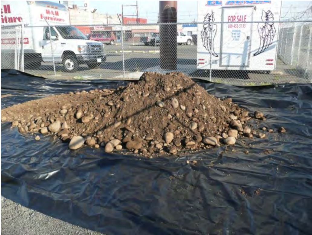
Photo 4 - Stockpiled spoils on lining. 4/24/12
