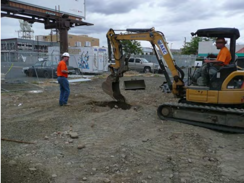
Photo 41 - AEC collecting confirmation samples of import material trench fill for chemical analysis. 5/22/12
