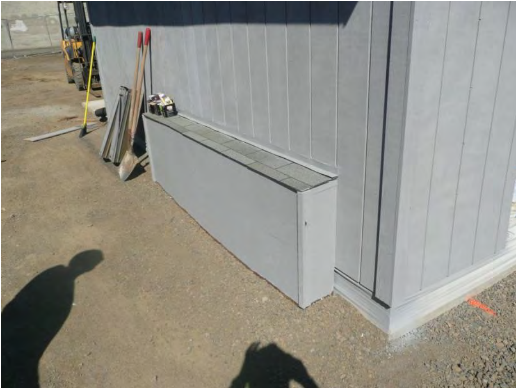
Photo 56 – Box extended to cover piping transition from above ground to below and protected with insulation inside. 6/14/12
