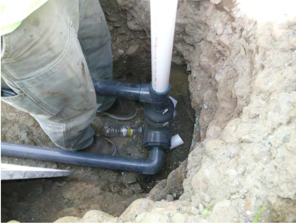
Photo 19 - SVE well pipe connection showing the lower zone 2-inch piping above and the upper zone 4-inch annular space piping below. 5/01/12
