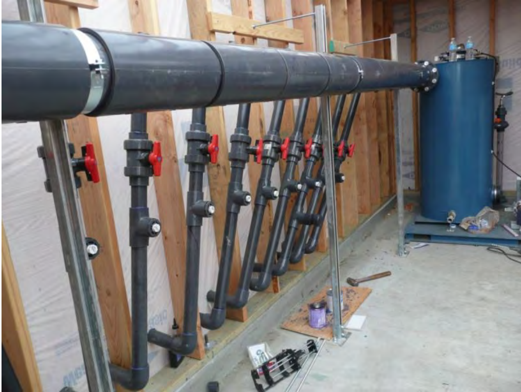
Photo 46 - SVE manifold and moisture separator. 5/31/12
