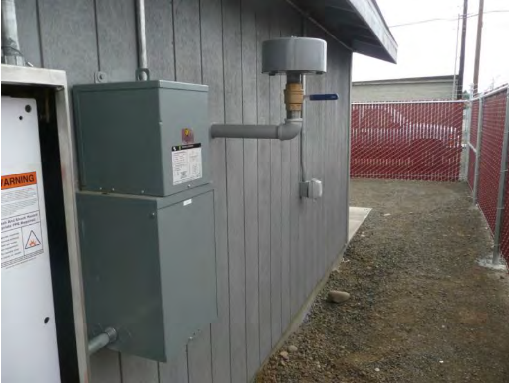
Photo 73 - Transformer and air dilution valve on exterior of SVE utility building. 7/12/12
