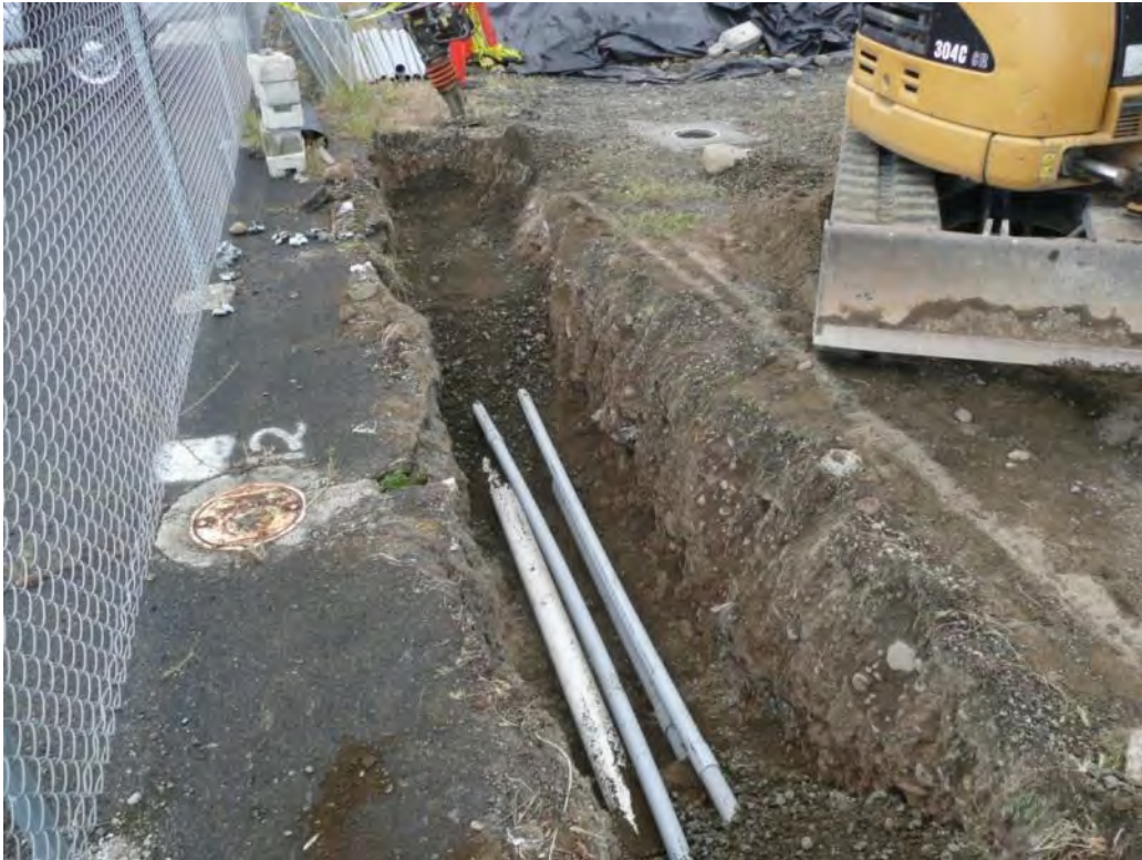
Photo 26 - Utility trench with 4-inch Schedule 40 PVC spare for future groundwater recirculation lines. 5/04/12
