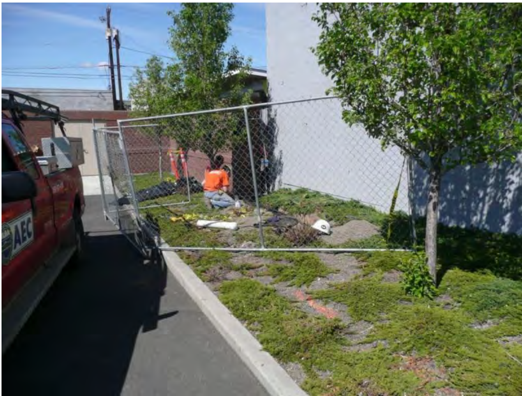
Photo 10 - Security fencing around SVE-3. 4/27/12
