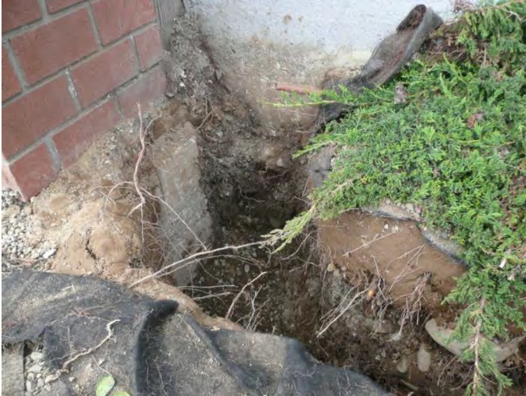
Photo 5 - Excavation by hand to SVE-3 on the southern side of the childcare center building. 4/25/12
