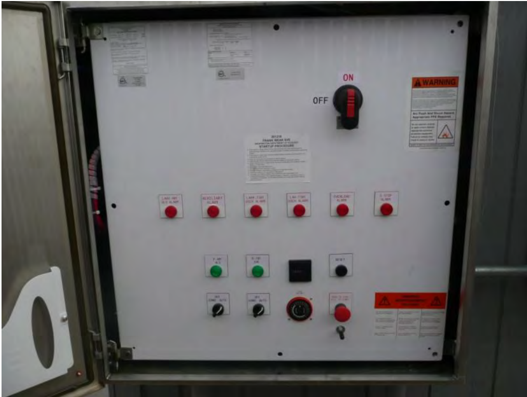
Photo 72 - Control panel located on exterior of SVE utility building. 7/12/12
