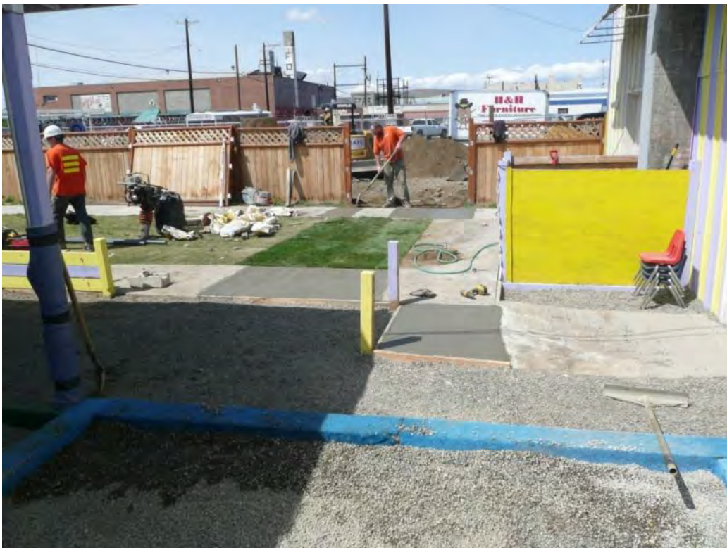
Photo 14 - Completed trench to SVE-3 with additional 4-inch PVC from wood fence and cored through concrete wall on south. 4/29/12
