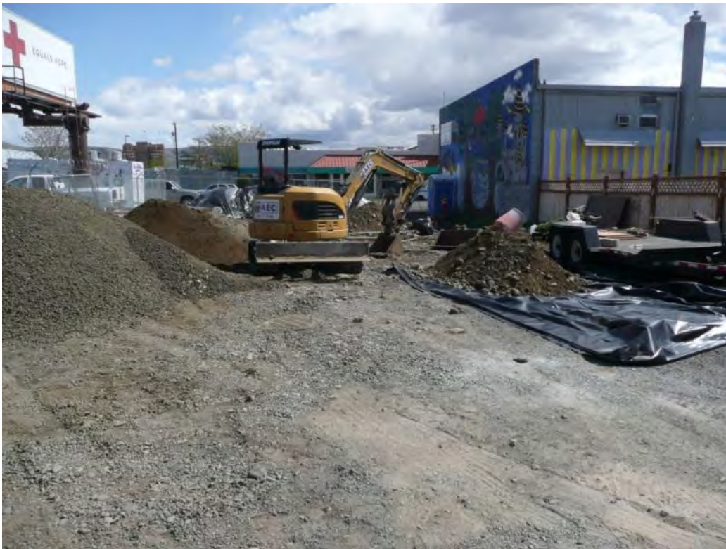
Photo 16 - Excavation for trenches to SVE-2, SVE-3, SVE-4, and SVE-5 completed. Spoils on lined and covered stockpiles. Imported beddings, sand and 1-1/4-inch backfill material onsite. 4/30/12
