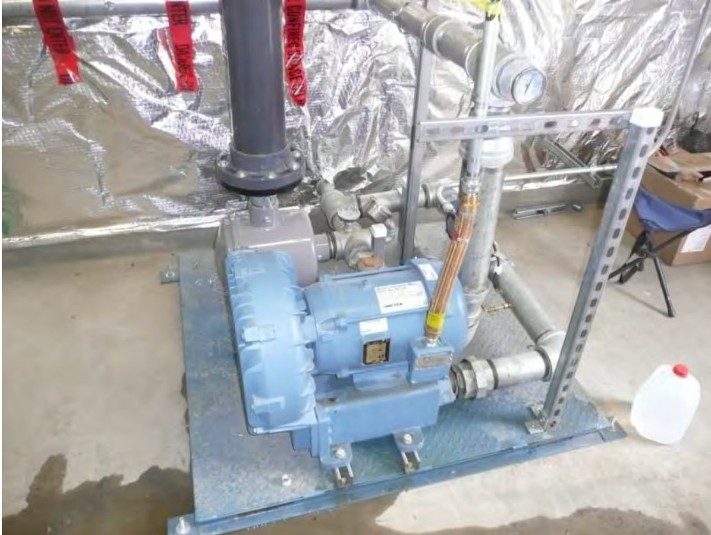
Photo 71 - SVE blower, inlet filter, and discharge temperature gauge. 7/12/12
