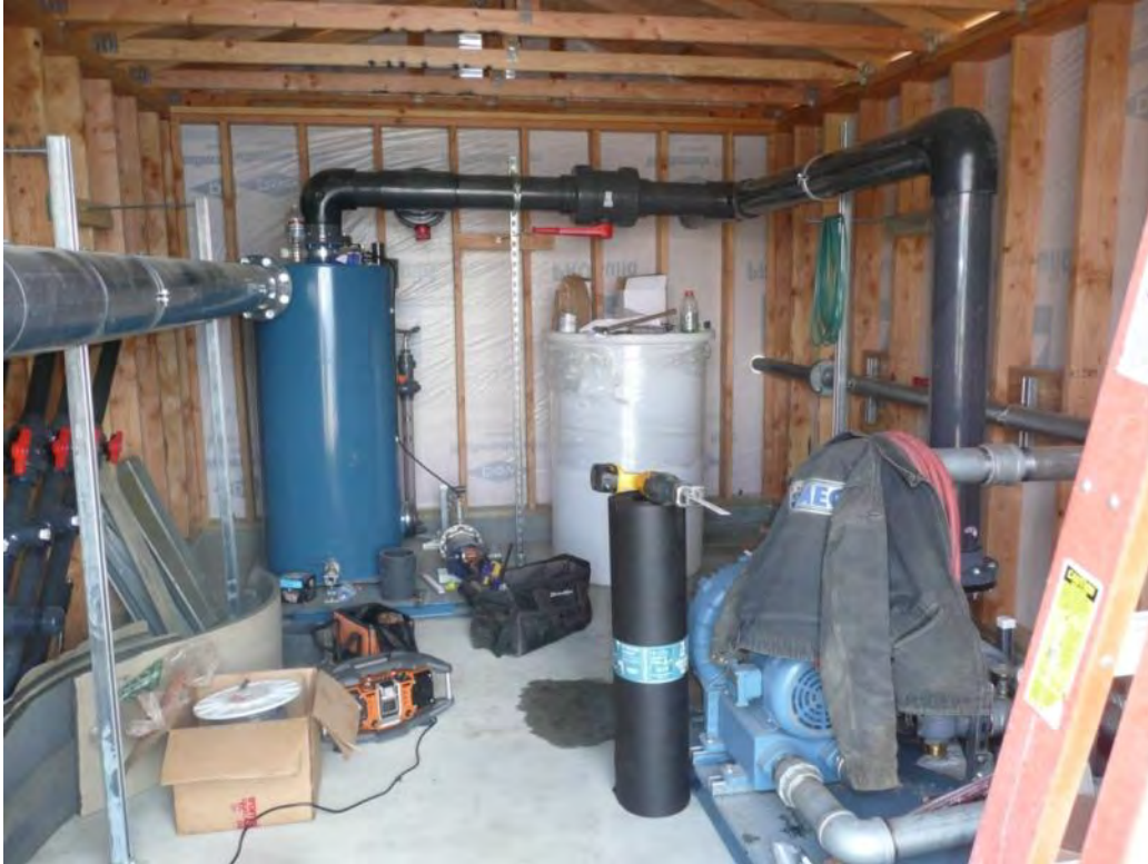
Photo 53 - Equipment and piping extent constructed inside SVE utility building. 6/07/12
