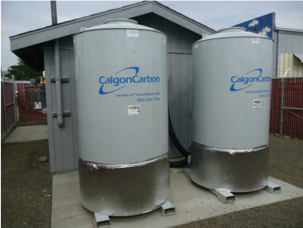
Photo 74 - GAC cans with insulation over heat trace. 7/12/12
