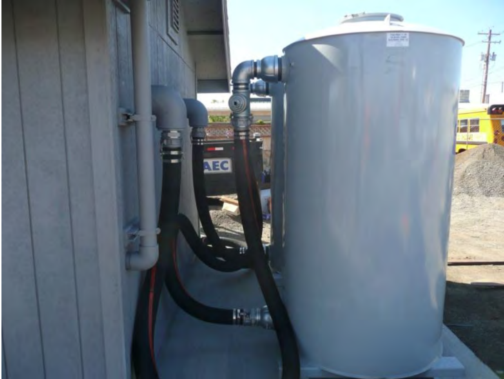
Photo 55 – GAC units position on concrete pad and connected. 6/14/12
