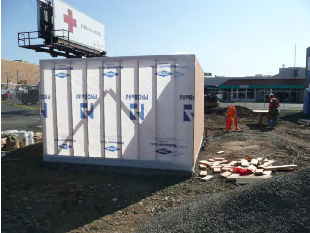
Photo 39 – SVE utility building with vapor barrier. 5/18/12
