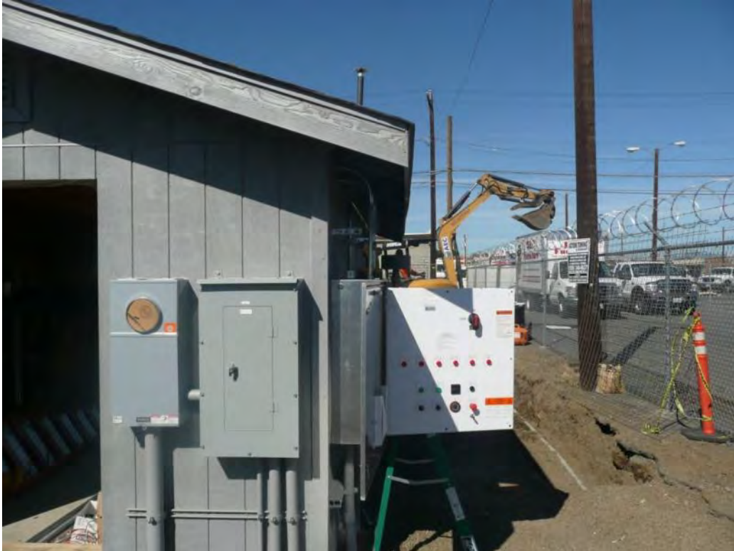
Photo 58 – Meter box, service panel, and SVE control panel. 6/15/12
