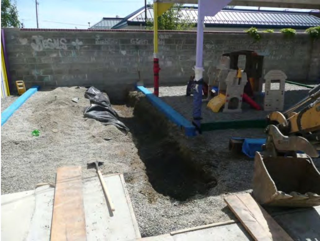
Photo 59 - Playground trench re-excavated to remove impacted 1-1/4-inch CSBC. Chemical analysis detected polycyclic aromatic hydrocarbons (PAHs) in previous confirmation samples. 6/15/12
