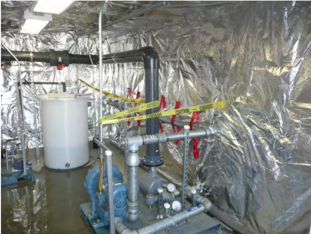
Photo 68 - Water in discharge tank after testing pump and floats on Vapor Liquid Separator (VLS). Caution tape and "HOT" labels on piping. 7/3/12
