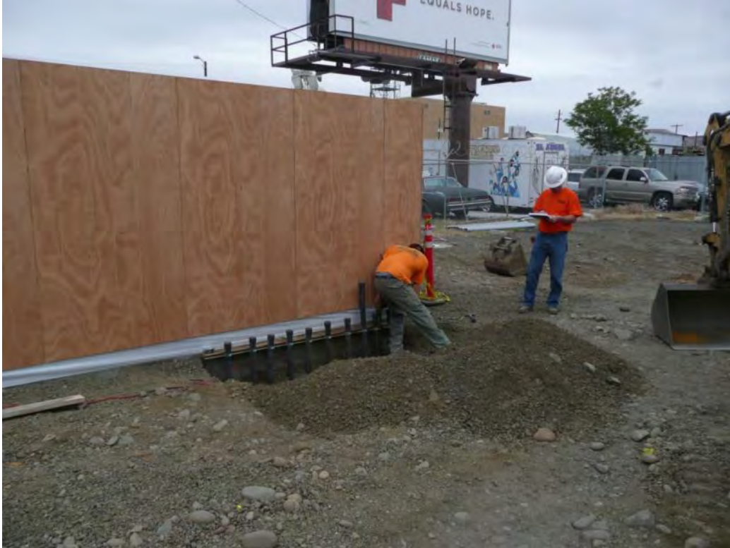
Photo 40 - SVE 2-inch piping spaced for utility building entrance and manifold. 5/22/12
