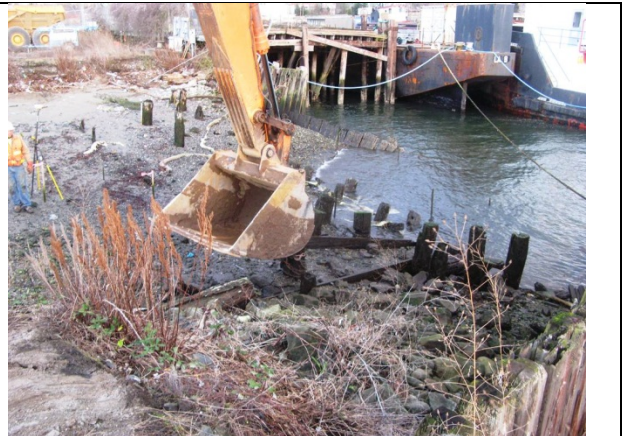
Comment: Attempting to remove/extract existing wood piling with Hitachi EX450 Excavator and chain choker.
