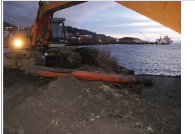
Comment: Wood pile extracted and staged at upland away from work area. Pile does not appear to be treated.
