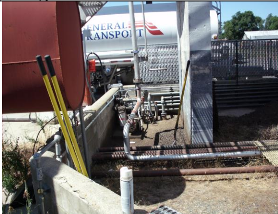
Photo #11: Soil staining on the north end of the split AST where the fuel spill occurred. Note secondary containment.
