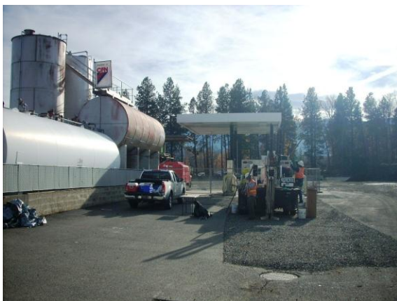
Photo #5: Borehole B-20 advanced to collect a groundwater sample in the previous excavated area south of the catch basin shown in the foreground. Photo looking south.
