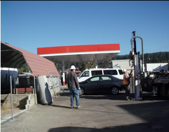
Photo #3: Location of borehole B-11 east of the aboveground fuel storage tanks area. Photo looking north.
