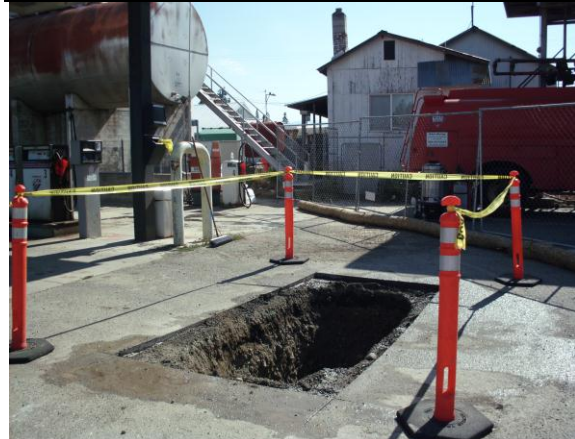
Photo #22: View looking northeast towards test pit south. Photo taken adjacent south of diesel fuel island w/canopy.
