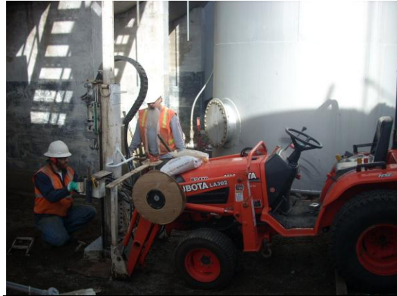
Photo #2: Direct push probe drilling at borehole B-16, adjacent south of split tank AST (fuel spill area) within containment. Photo looking north.
