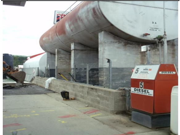
Photo #12: Photo showing the west side of the AST enclosure and the diesel fuel dispenser pump. Looking north-northeast.
