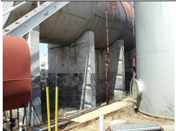
Photo #10: Area of fuel spill beneath the split aboveground storage tank (AST).
