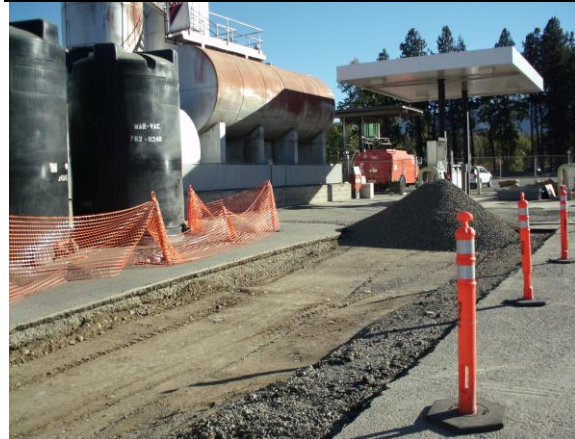
Photo #24: Backfilled excavations of the main test pit comprising of test pits TPN and TPN2.
