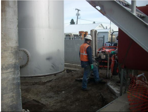
Photo #1: Limited access rig advancing borehole B-18 within southeast area of bulk fuel containment area. Photo looking northeast.
