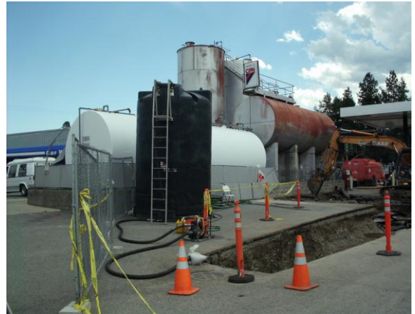
Photo #14: Photo of the AST enclosure looking southeast. Note poly tank in foreground and pump for groundwater seepage within test pit north excavation.
