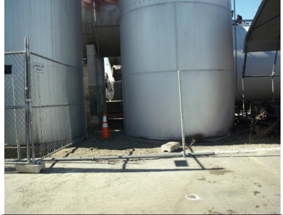
Photo #8: Location of borehole B-7 shown in white paint east of the diesel fuel aboveground storage tank (in the background). Photo looking west
