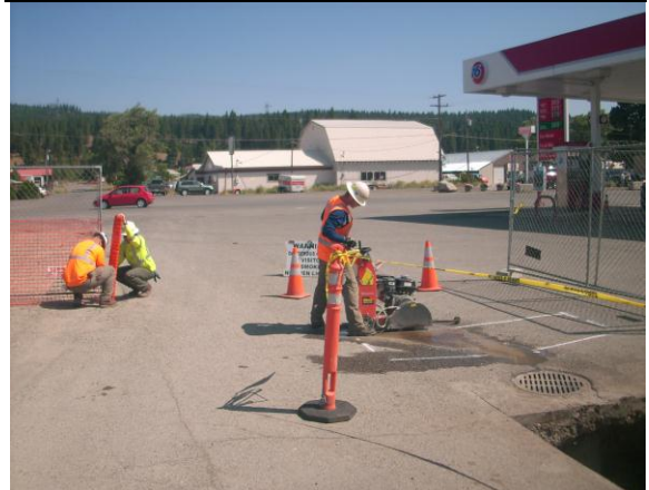
Photo #18: View looking north-northeast at initial asphalt cutting in preparation of test pit north 3.
