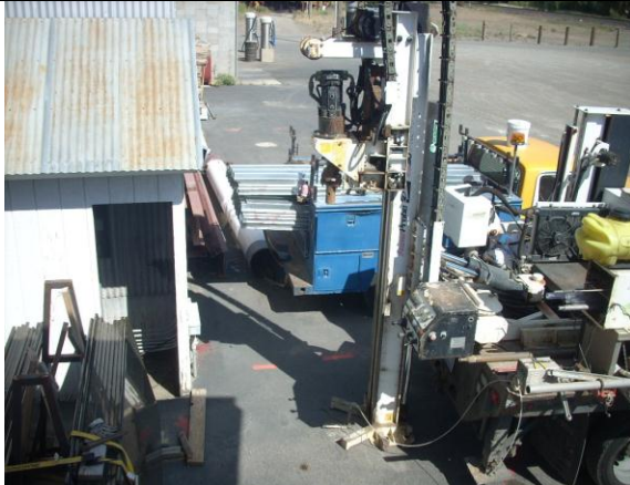
Photo #11: Location of borehole B-9 on the southwest corner of the office building. Photo looking southeast
