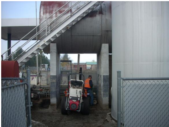
Photo #3: Borehole B-17 advanced beneath the split tank AST within bulk fuel containment area. Photo looking west.
