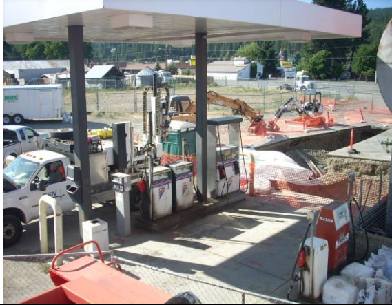
Photo #7: Borehole B-6 advanced within the diesel dispenser area, southwest of the aboveground storage tanks and south of the test pit excavation. Photo looking northwest
