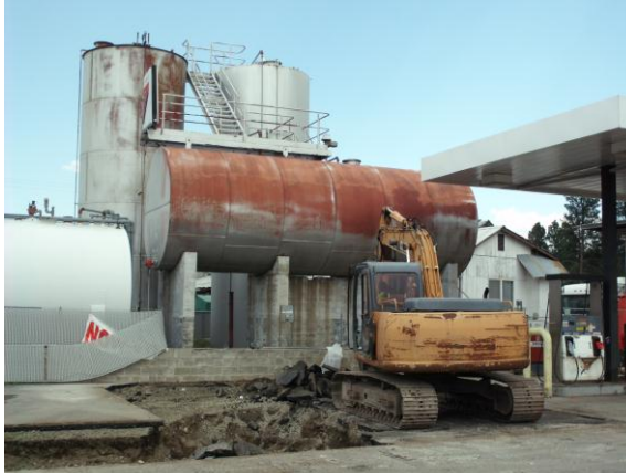
Photo #15: View looking east-southeast toward the initial excavation of test pit north 2, located adjacent west of spill location.
