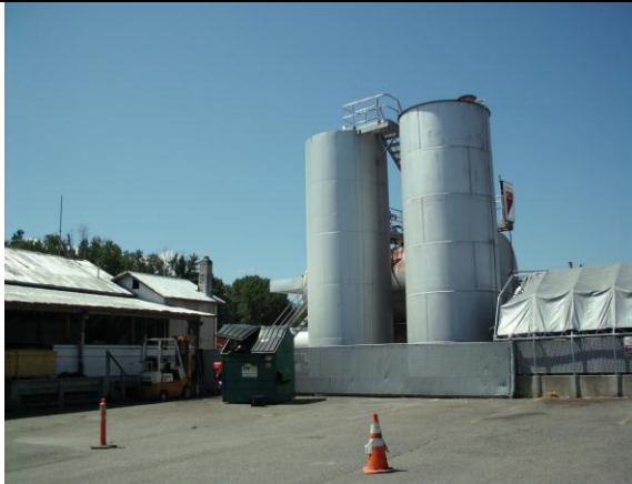
Photo #3: View looking southwest at eastern side of ASTs fuel farm where spill occurred.
