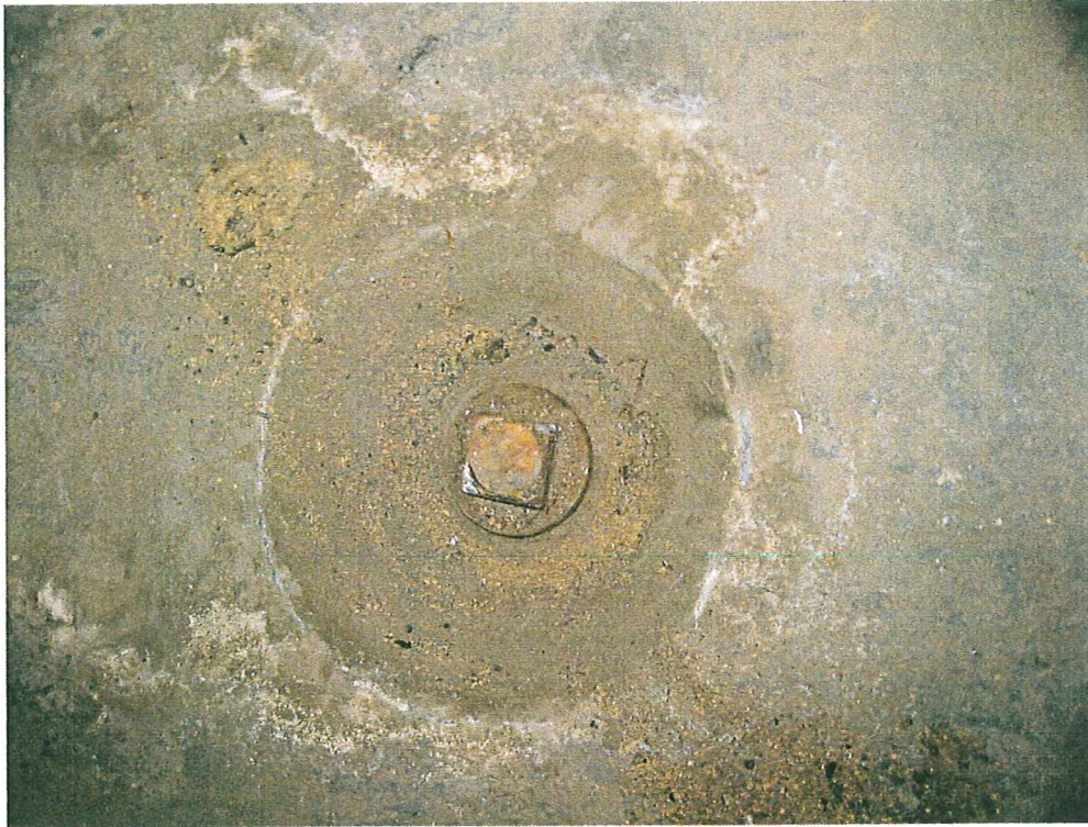
UST fill port, Substation building.
