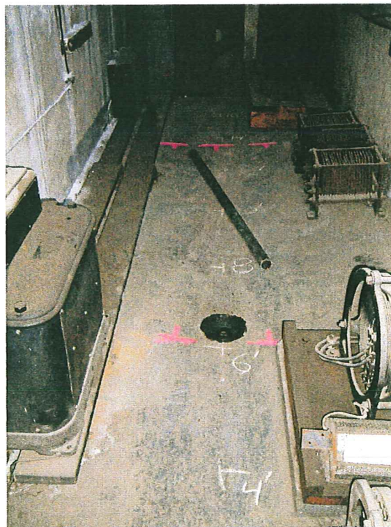
UST in Substation building with location/length marked based on GPR survey.
