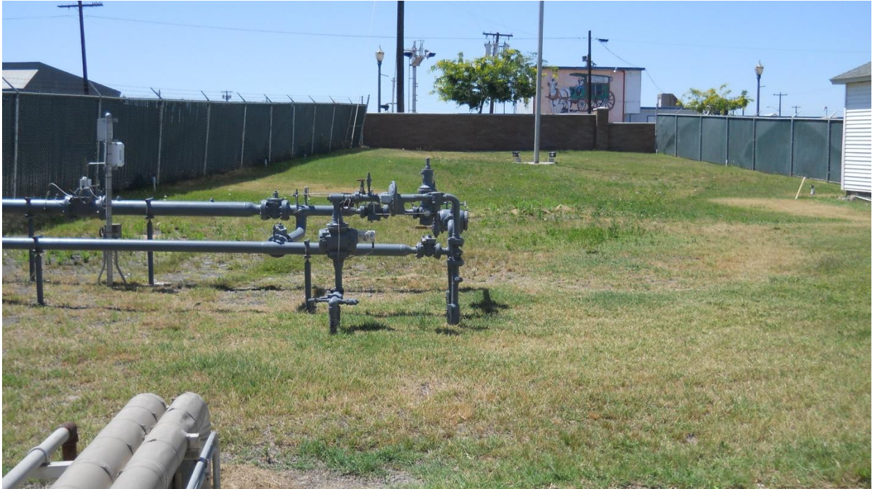
Figure 6. Photograph of Area Where Underground Storage Tanks Were Removed. (Looking to the West)
