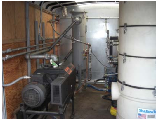
Busch Vacuum Pump (front left) , Knock Out Chamber (back left) and Air Stripping Tower (front right)
