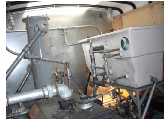
Knock Out Chamber and Oil Water Separator
