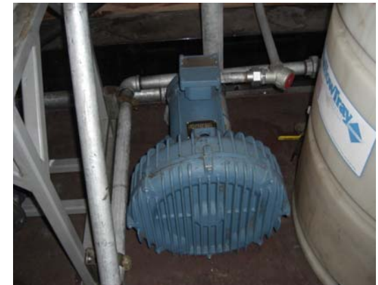
Air Stripper Blower
