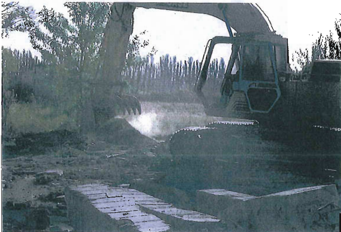
Photo 8 Demolition of hop picker building completed at 3:45pm Monday, October 4, 2004. Demolition of NE corner of former hop picker building foundation begins October 5, 2004. Demolition of the NE corner foundation takes approximately 40 minutes to complete.
