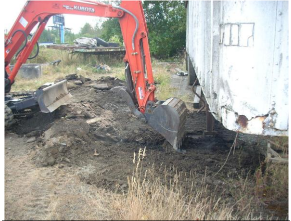
Photo #2: View of petroleum stained soil being excavated and location of soil sample EX1-1 & EX1-1.5.
