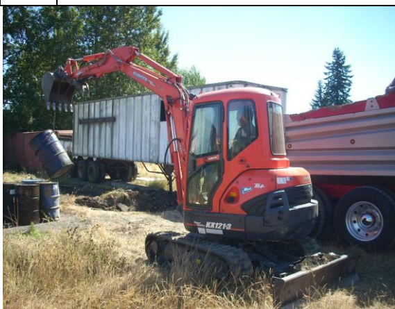
Photo #11: View of onsite drums being loaded into dump truck for removal.
