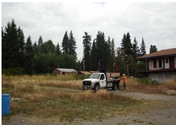
Photo #5: Direct push probe drilling at boring B-2 on Parcel B in vicinity of diesel fuel spill and former auto wrecking yard. View looking northwest.
