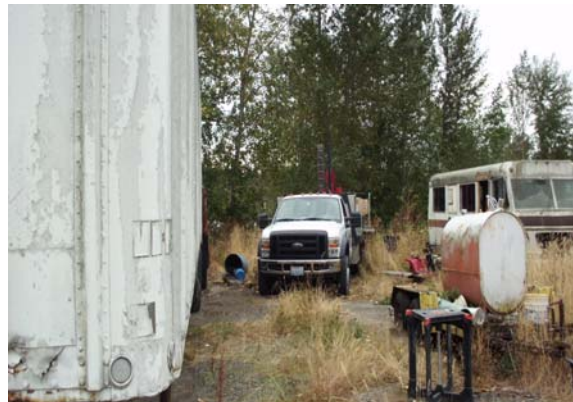
Photo #4: Direct push probe drilling at boring B-4 in southeast portion of Parcel A where stains on ground and unlabelled containers and 55 gallon drums were documented. View looking east.
