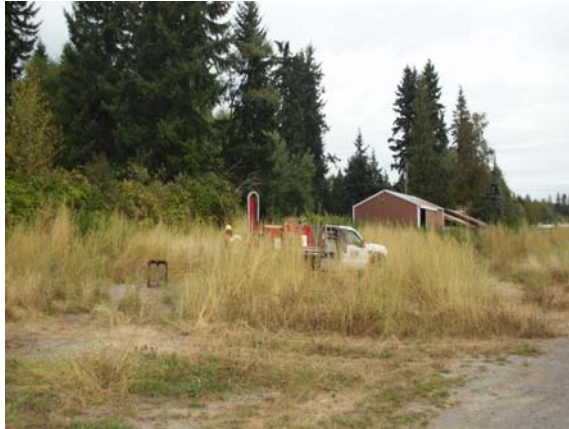
Photo #7: Direct push probe rig at boring B-7 in west central Parcel C. View looking north.
