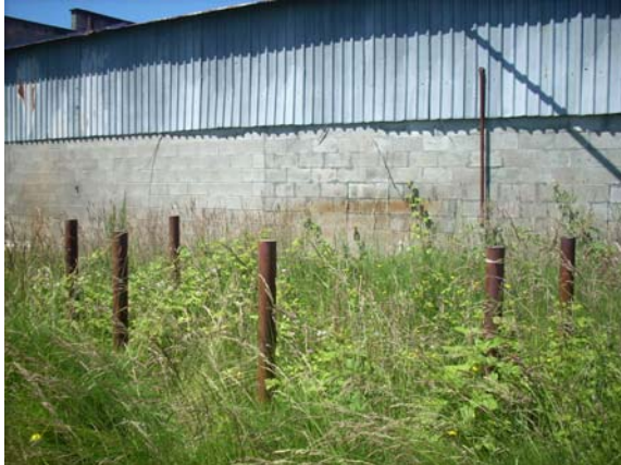
Photo #27: Location of suspected AST on southeast side of main auto body repair shop on Parcel A.
