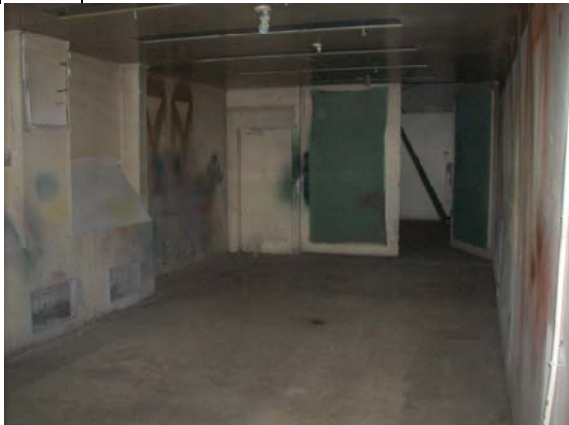
Photo #5: View of painting room on southeast side of main auto shop. Note air vents on far left.
