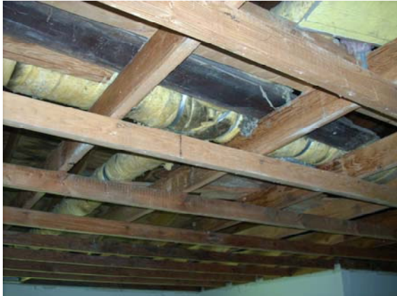
Photo #21: View looking at exposed ceiling in living room of Parcel C house.
