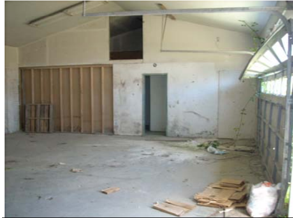
Photo #8: View of bay within minor auto shop and two smaller rooms and a bathroom through the hallway on the southeast side of the bldg.
