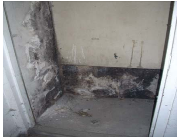
Photo #2: View of what appears to be a storage room on southeast corner of the main auto shop. Note drain in the center of the floor and extensive molding.
