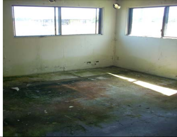
Photo #20: Representative view of condition and use of Parcel C house. Note extensive molding.
