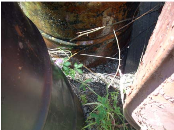
Photo #17: View of stained soil from overflow of drum (closest drum, photo 16). Overflow likely due to infiltration of rainwater.
