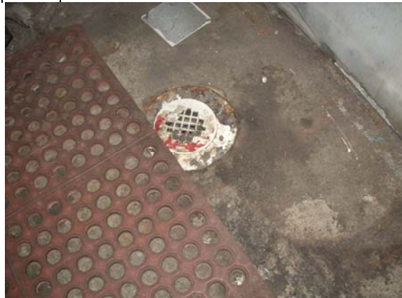
Photo #6: View of drain in what appears to be a cleaning/shower room on southeast corner of main auto shop.
