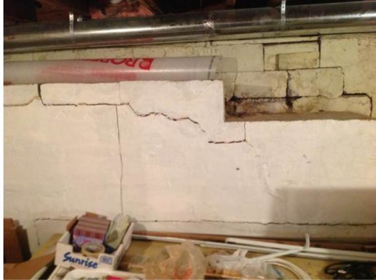
Photograph 21. Foundational cracks in the walls of the basement at 305 N 1st Avenue, July 2013.
