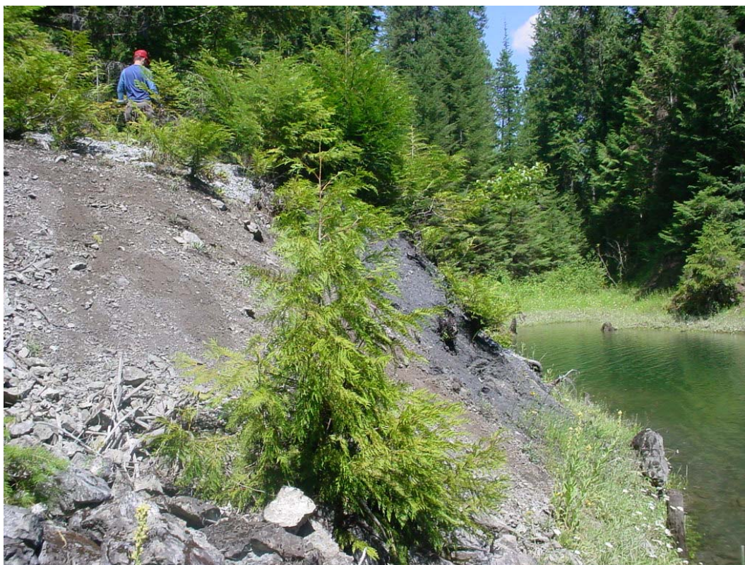
Photograph 1 - WR-1: Zone 1 (black material on right slope), Zone 2 (brown material on facing slope), and Zone 3 (gray material on top).
