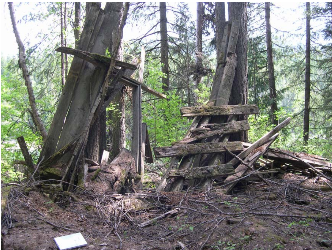
Photograph 5 - View of collapsed structure at east end of DB-1.
