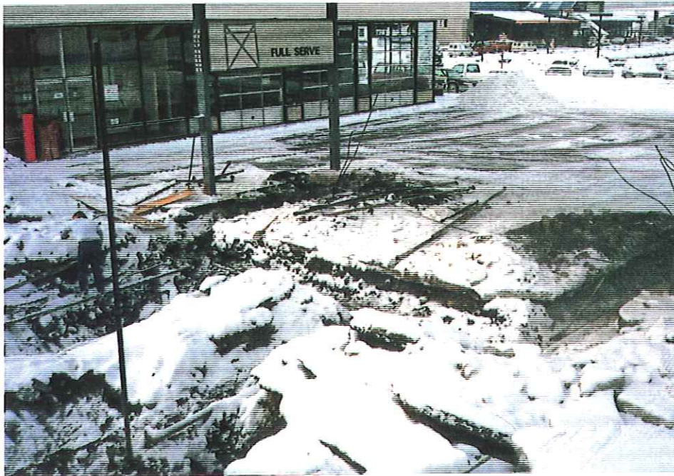
Site View Showing Pump Island and Lines
