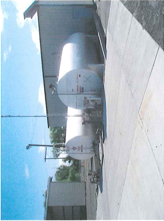
Jet A Fuel Aboveground Storage Tanks
