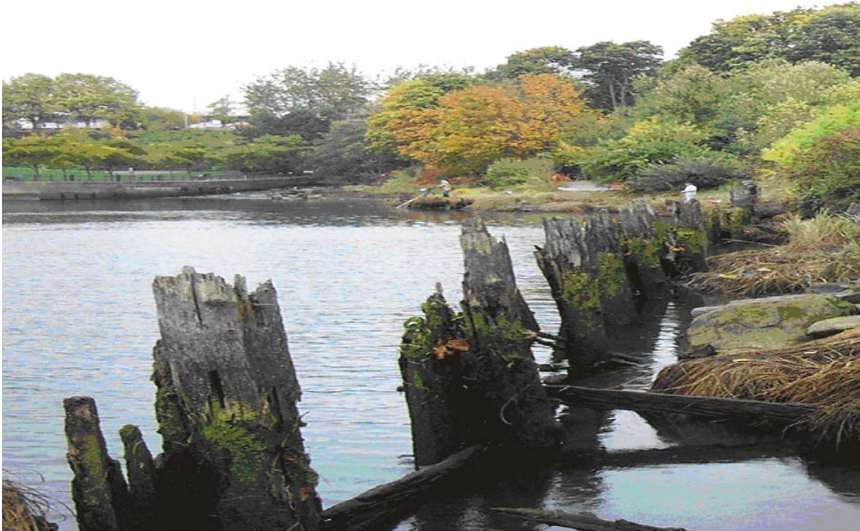
Photo 5-2. View of the south shoreline section containing a failing wood bulkhead.
