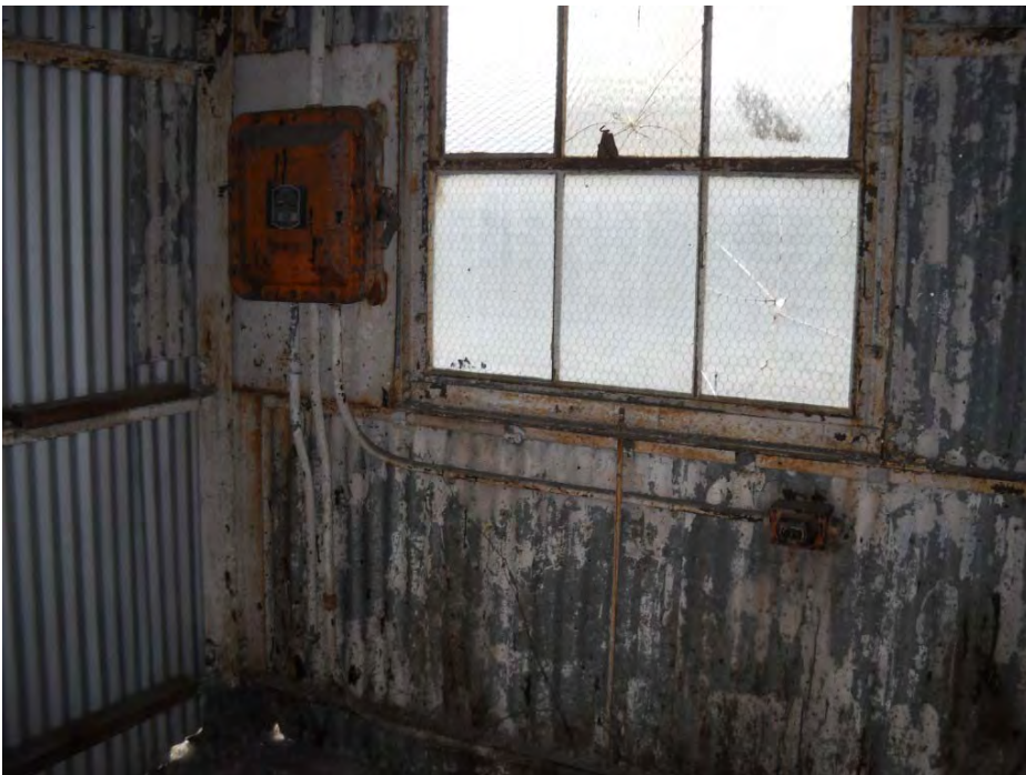
HSA No. 4. Electrical wiring (in electrical panel and conduit) (M)
