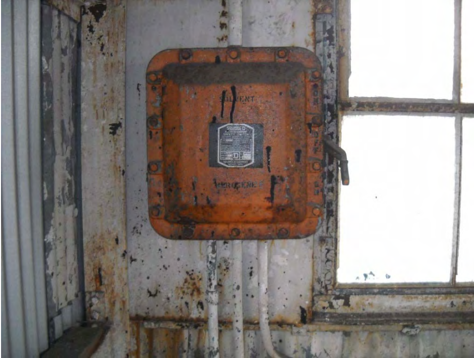
HSA No. 3. Electrical panel (M)
