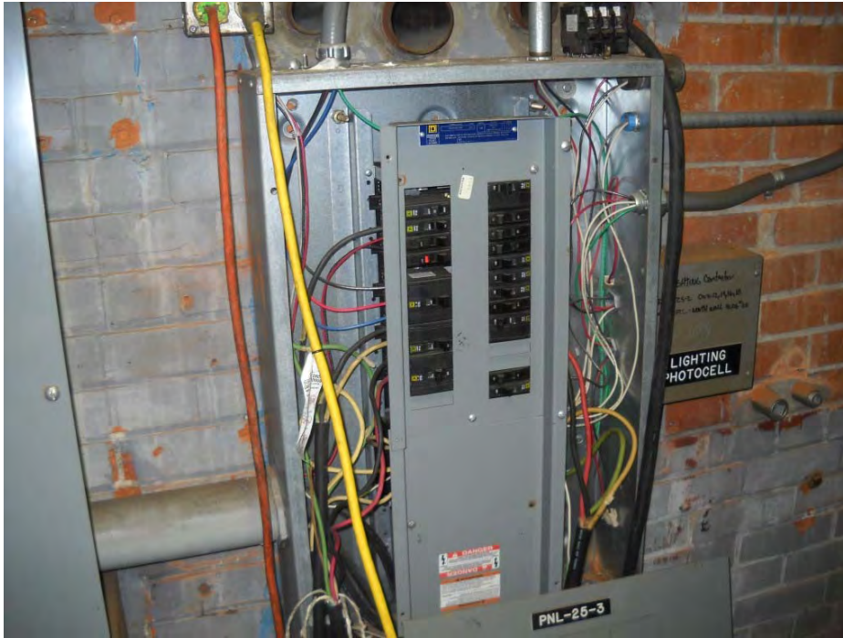
HSA No. 33. Newer electrical panels (M)
