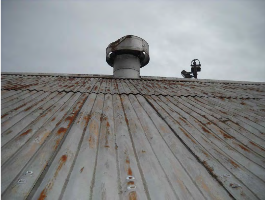
HSA No. 17. Silver paint and trace powdery material (M)
