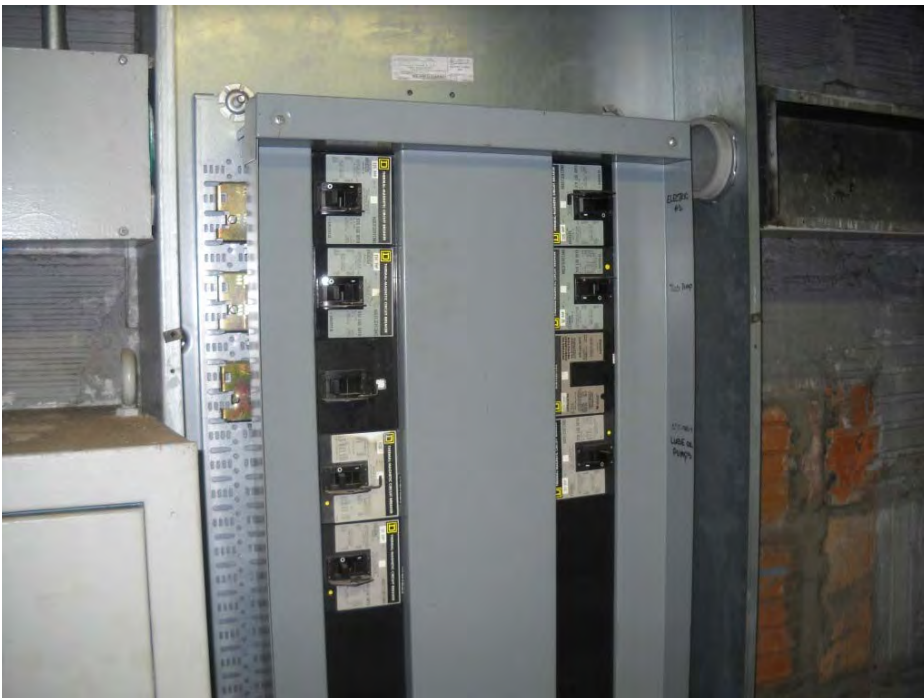
HSA No. 32. Large electrical panels and wiring (M)
