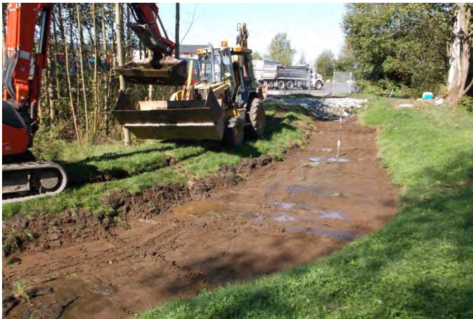
Photo 3. Excavated material was placed in a backhoe for removal from the site.
