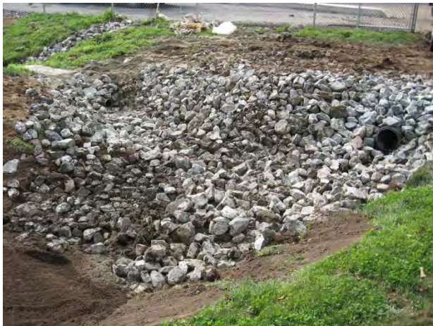
Photo 7. Rock was removed and replaced at the upper end of the bioswale below the inflow pipes.
