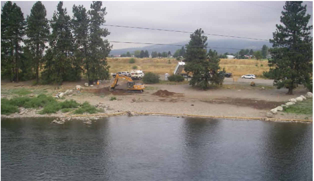
View of the site from the Harvard Road Bridge facing northwest during construction.
