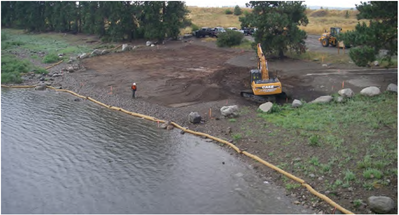
View of the site from the Harvard Road Bridge facing northwest during construction.
