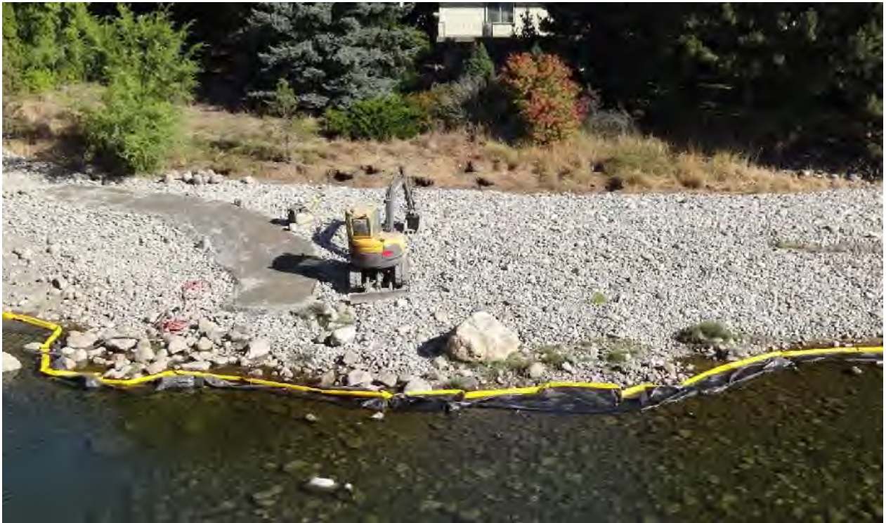
View of site from Barker Road North bridge facing north during construction.
