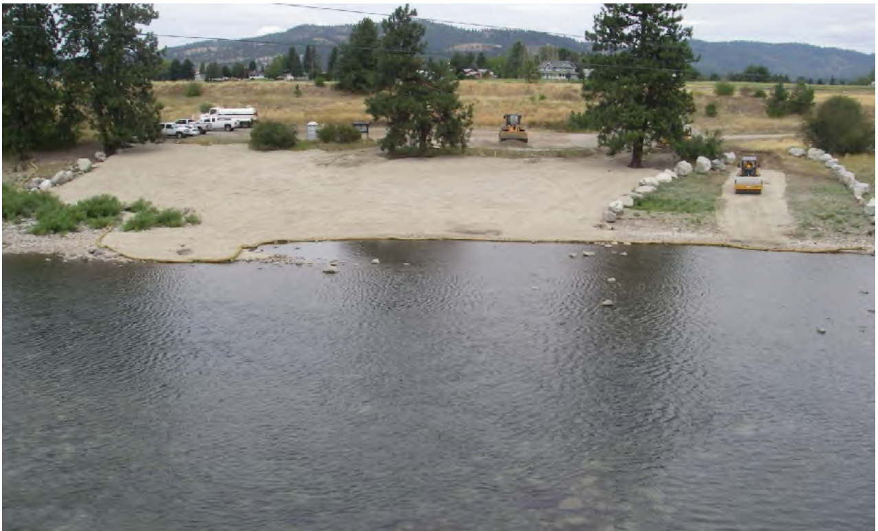
View of the site from the Harvard Road Bridge facing northwest during construction.
