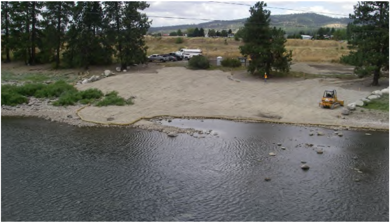
View of the site from the Harvard Road Bridge facing northwest during construction.
