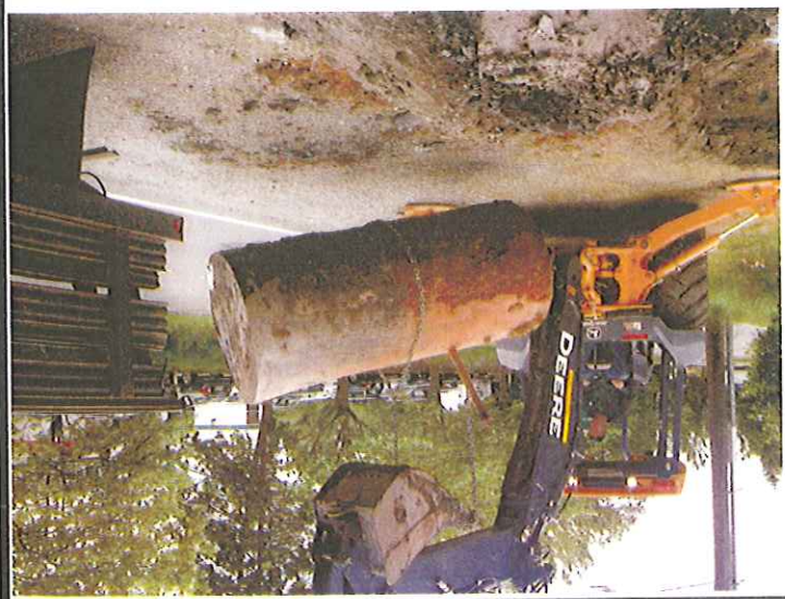
UST removed from the ground and loaded onto truck for off-site disposal.
