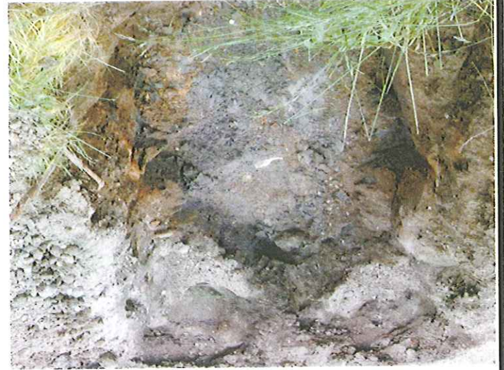
Excavation following UST removal. Exposed soils exhibiting gray-discoloration and moderate petroleum-odor. Groundwater seepage observed in side walls of excavation.
