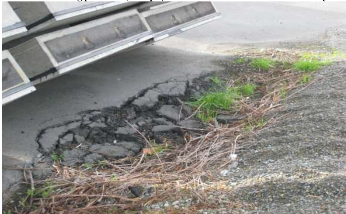
Photo 4: Deteriorating pavement (example) not near contamination – from the entry
