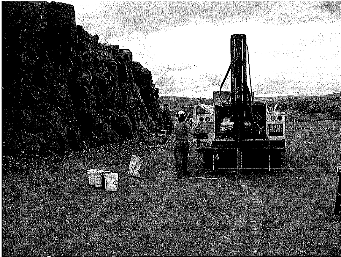
Photo # 3 Before – Geoprobe machine sitting on cover of disposal site and operator indicate scale of basalt outcrop bluff which forms south wall of bowl in which the disposal site sits. (Photo by Jeff Newschwander)
