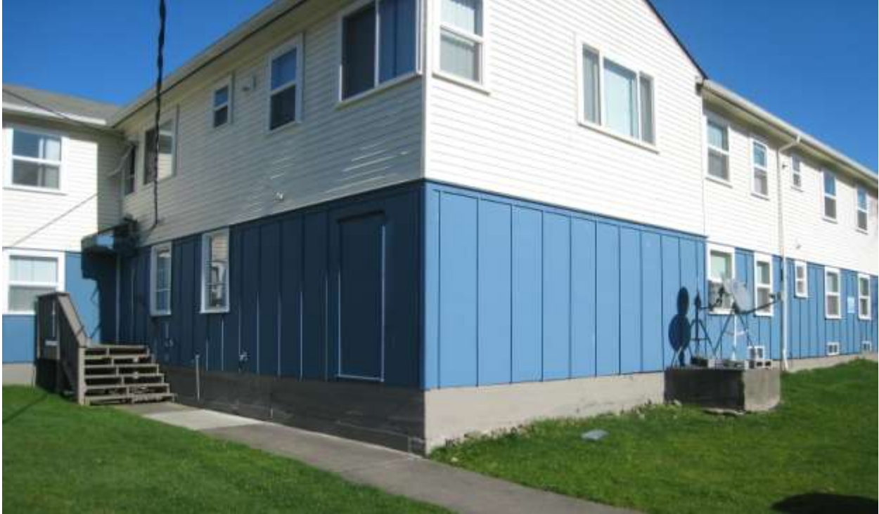
Photo 3: Typical location of tanks removal and excavation– concrete blocks at all locations
