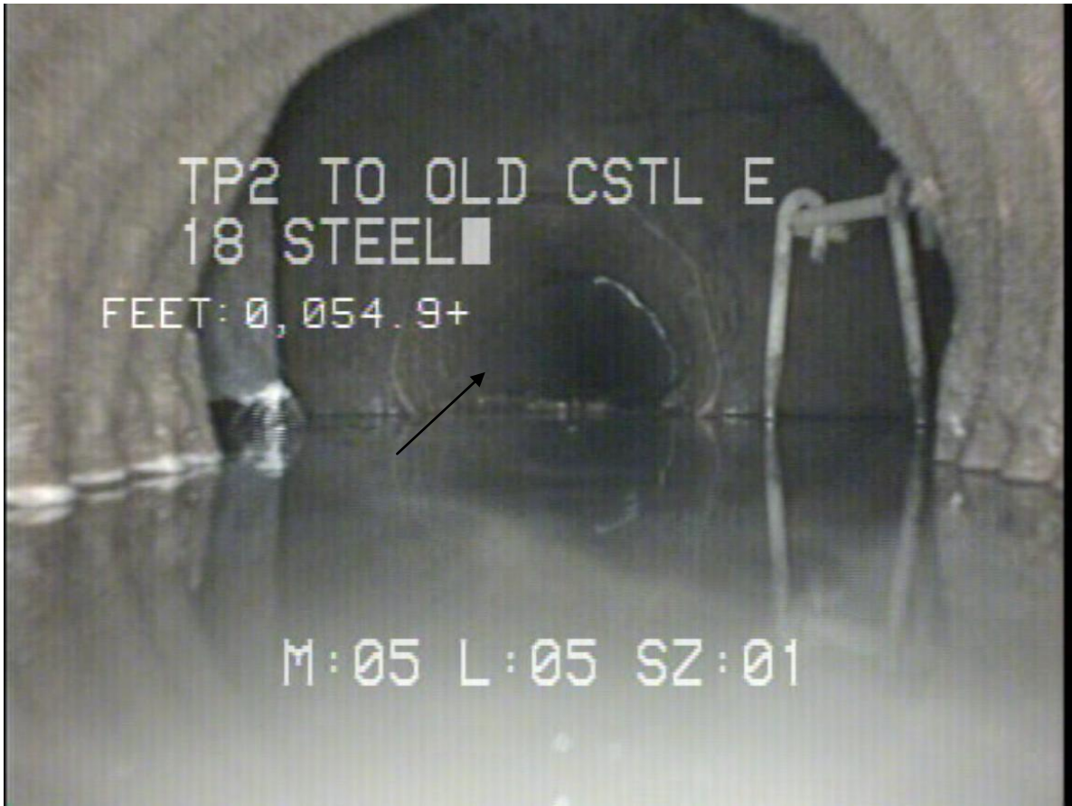
Photo 5. Deformation of CMP observed during video survey completed following the 2008 pipe failure. Arrow indicates area where pipe appears to be crushed.
