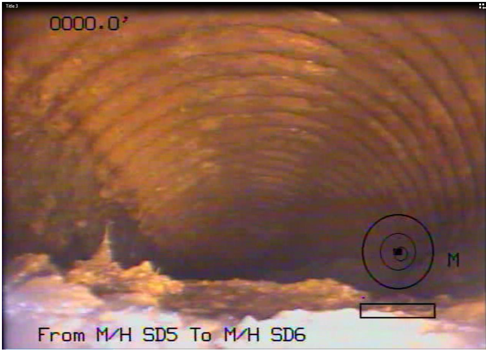
Photo 1. Contents of trunk line between catch basins SD-5 and SD-6.
