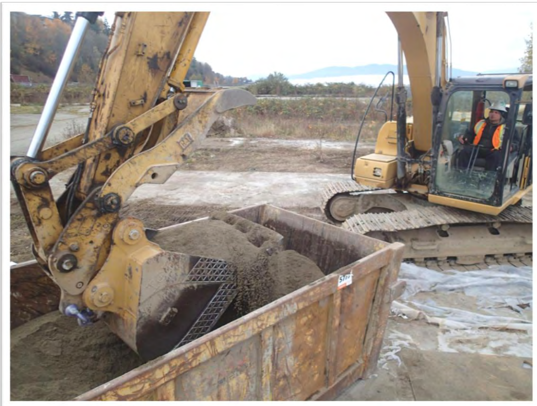
Photo 5: Mixing sand and organoclay on site to prepare amended cap (50/50 sand organoclay mix)
