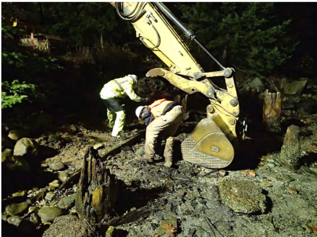
Photo 4: Removal of debris and large rocks from the Interim Action Area to prepare mudline for cap placement
