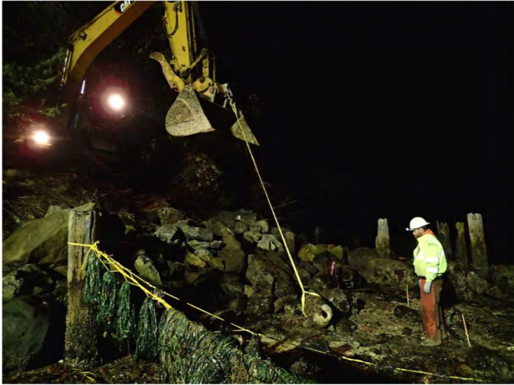
Photo 3: Removal of derelict wood piles from the Interim Action Area to prepare mudline for cap placement
