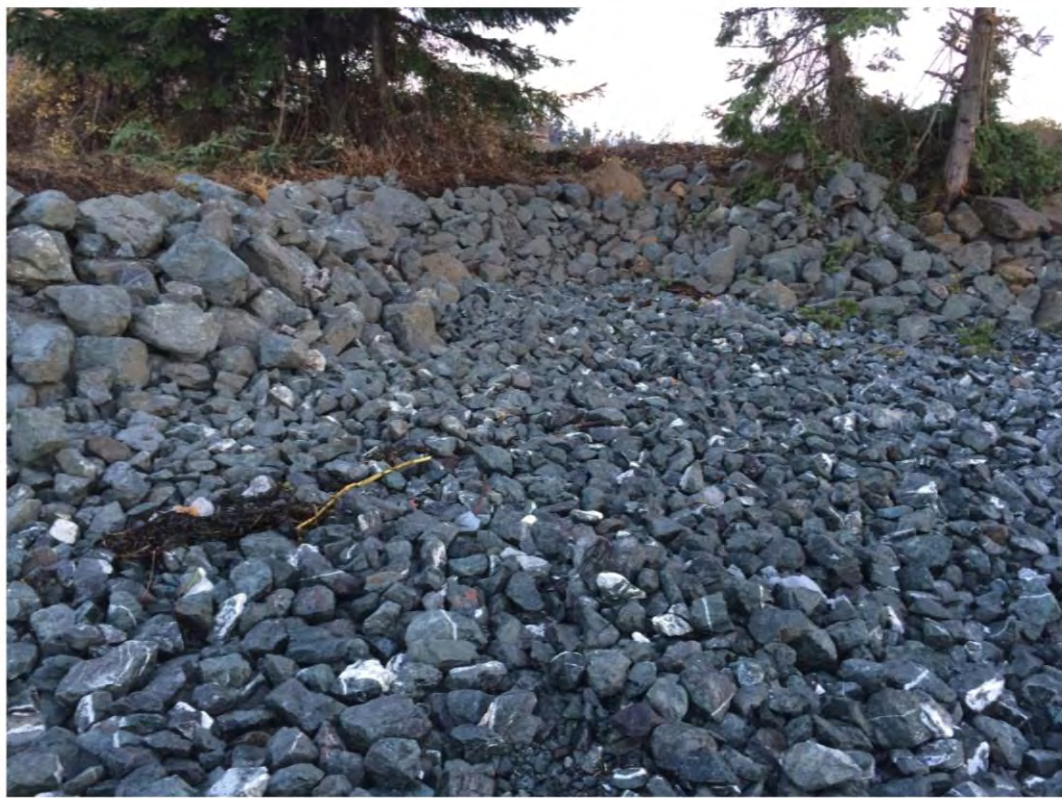
Photo 12: As-Built conditions of sediment cap and riprap placed during the Interim Action
