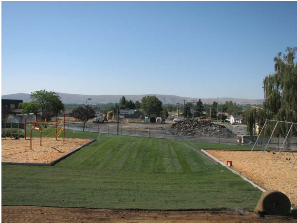
Photo D-9: Apple Valley Elementary School playground area; parking lot construction in progress.
