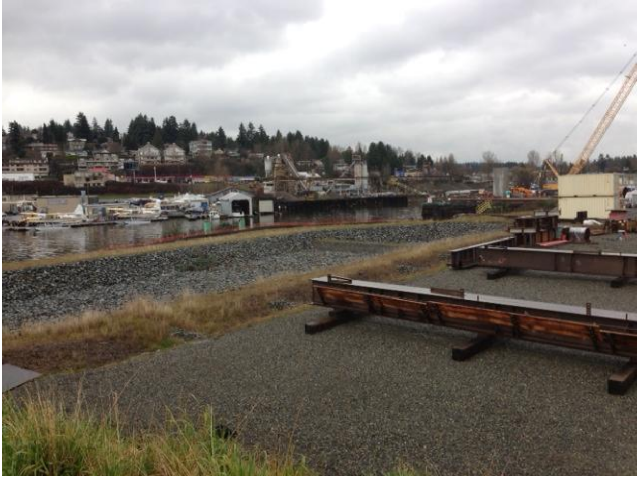
Appendix E -2. KIP Site at northwest corner gravel surface work area, storm water drainage basin, and Navigation Channel looking northeast.
