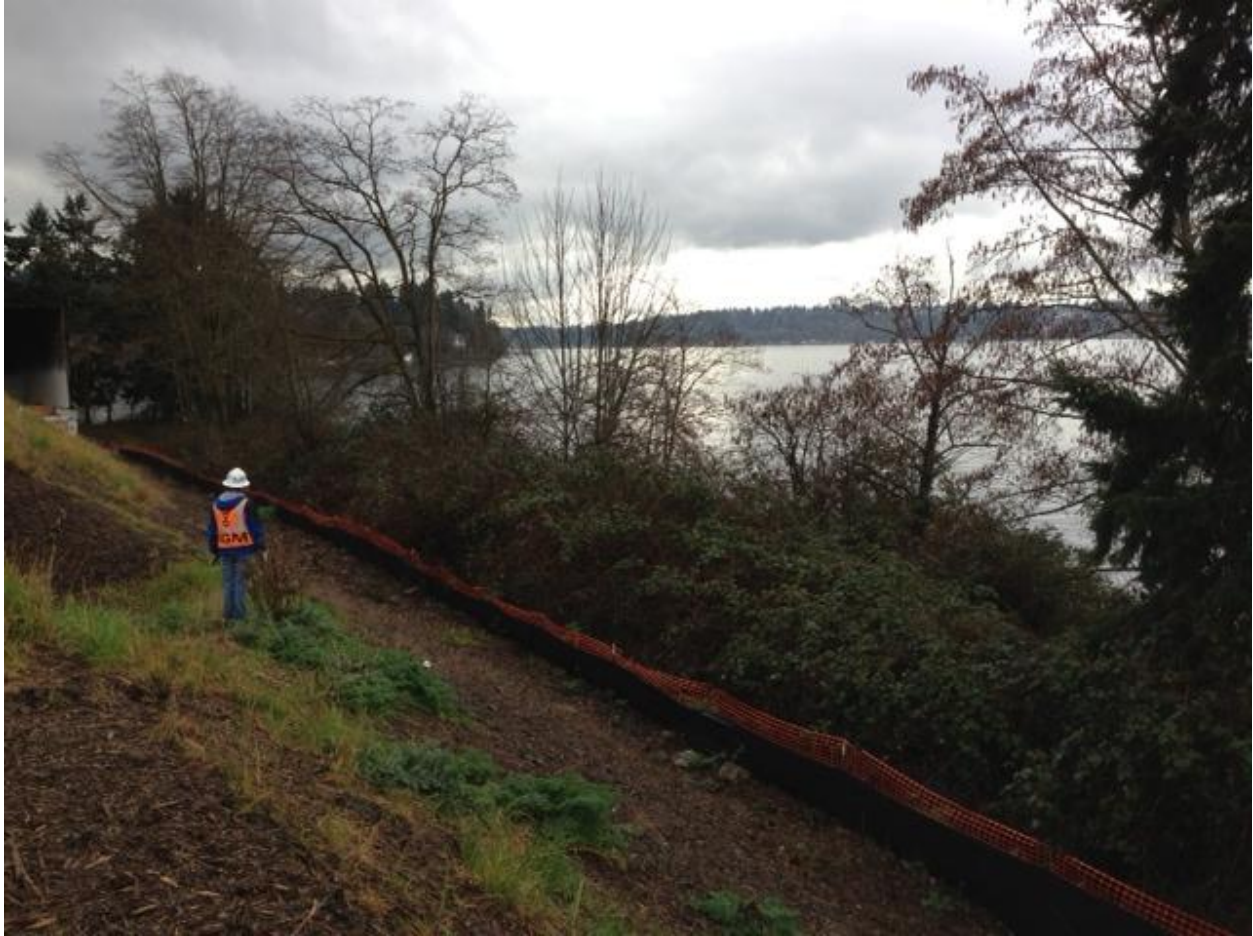
Appendix E -3. KIP Site at west side looking southwest to Lake Washington where worker is standing on berm, fence below (black and orange) and Wetlands A described as a class 2 palustrine forested/scrub-shrub wetland located at the west shoreline at Lake Washington (AMEC 2001 and Beak Consultants Inc. 1997).
