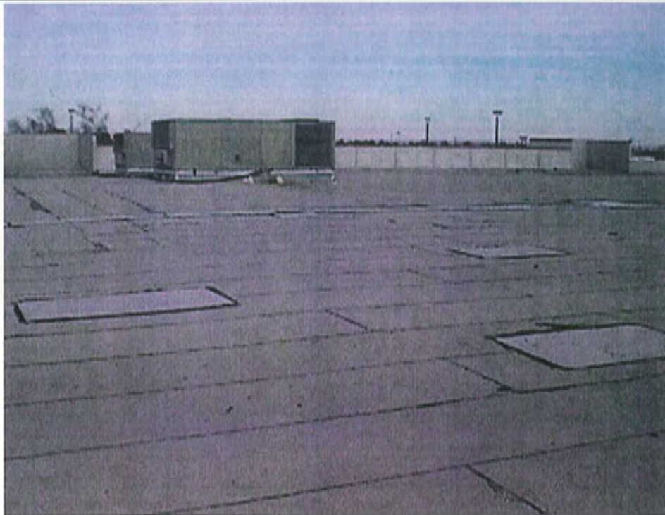
Photo 9: View looking southeast across the roof of the former Ernst store. Asbestos cement sheet material board is on the parapet wall in the background.
