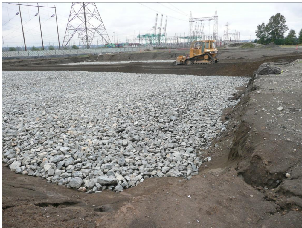
8. Looking southwest across the Closed Landfill area after placement of quarry spalls and during placement of surficial sand fill material.
