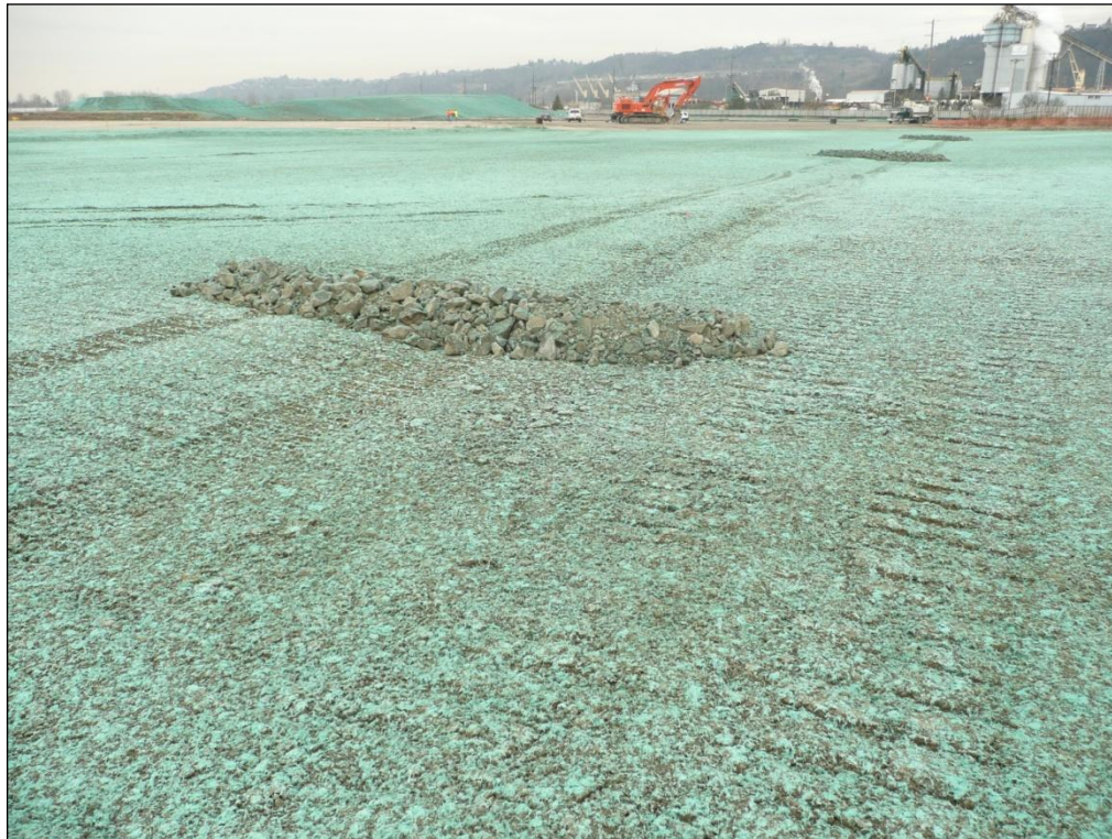
9. Looking northwest at the quarry spill check dams placed across the central drainage swale after completion of excavation backfilling.
