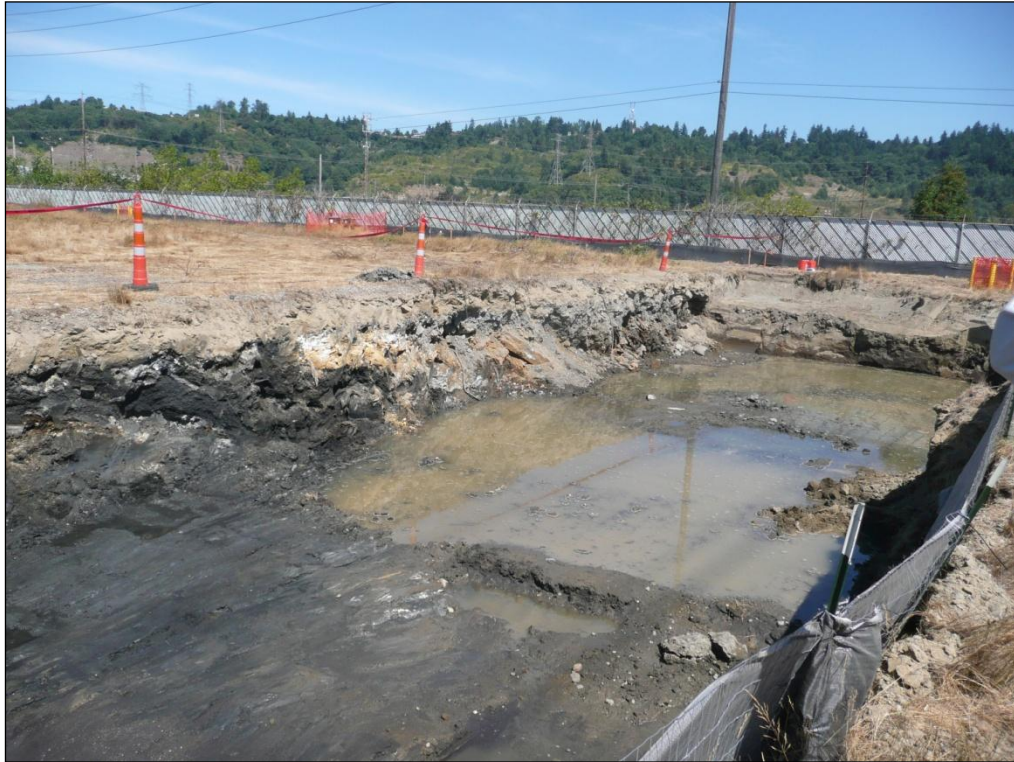
1. Looking northeast from the southern side of the Closed Landfill excavation (in progress).
