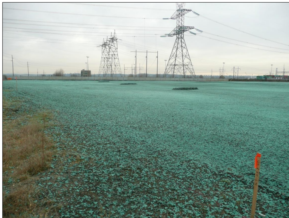
10. Looking southwest across the Closed Landfill area after completion of excavation backfilling and hydroseeding.
