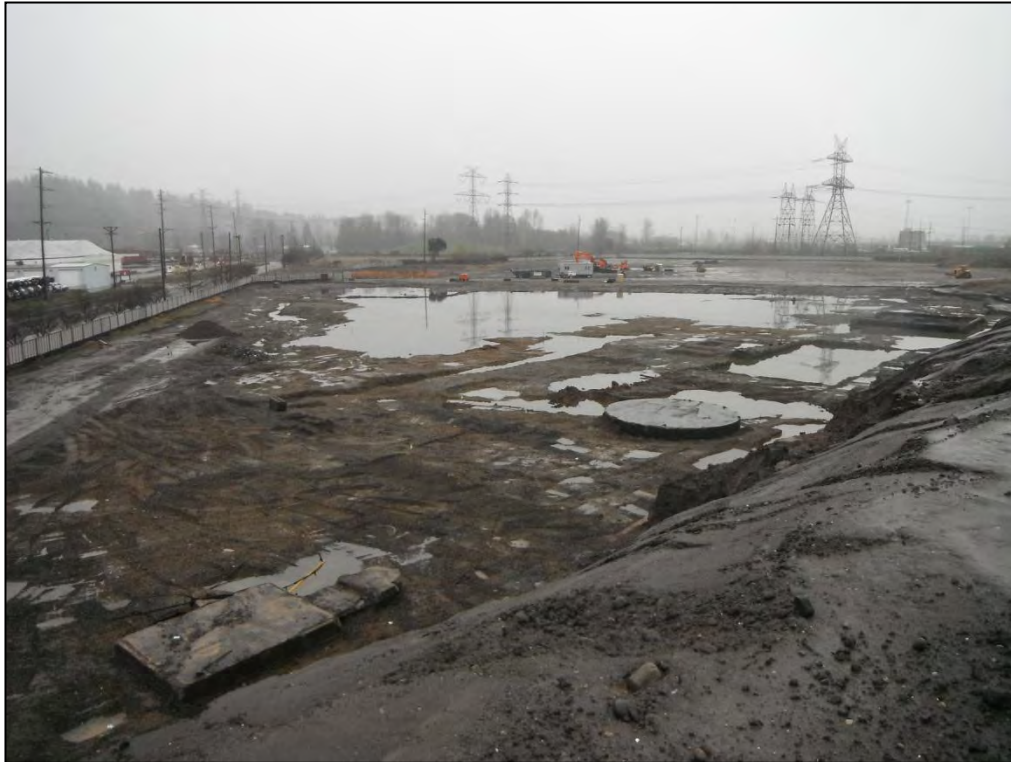
15. Looking southeast across the completed SPL Area excavation from the dredged soil stockpile, with water ponded in a significant portion of the excavation.
