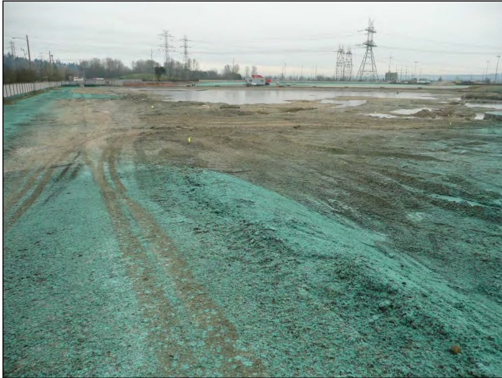
17. Looking southeast across the completed SPL Area excavation from the northern end of the dredged soil stockpile.
