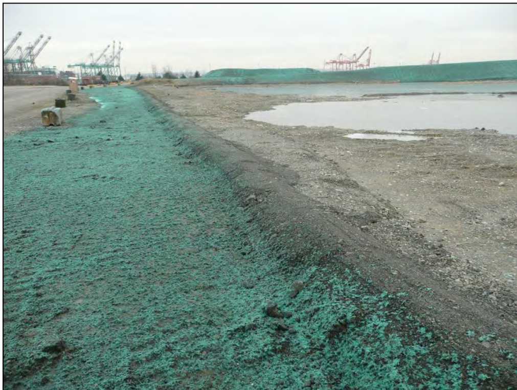
16. Looking southwest at the stormwater diversion berm constructed along the south side of the SPL Area excavation where water is ponded.
