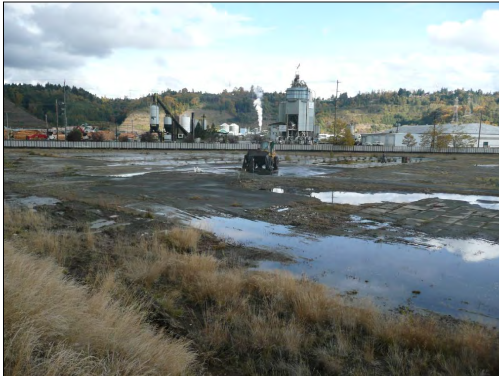
1. Looking northeast across the SPL Area prior to removal of surficial concrete slabs and asphalt pavement.
