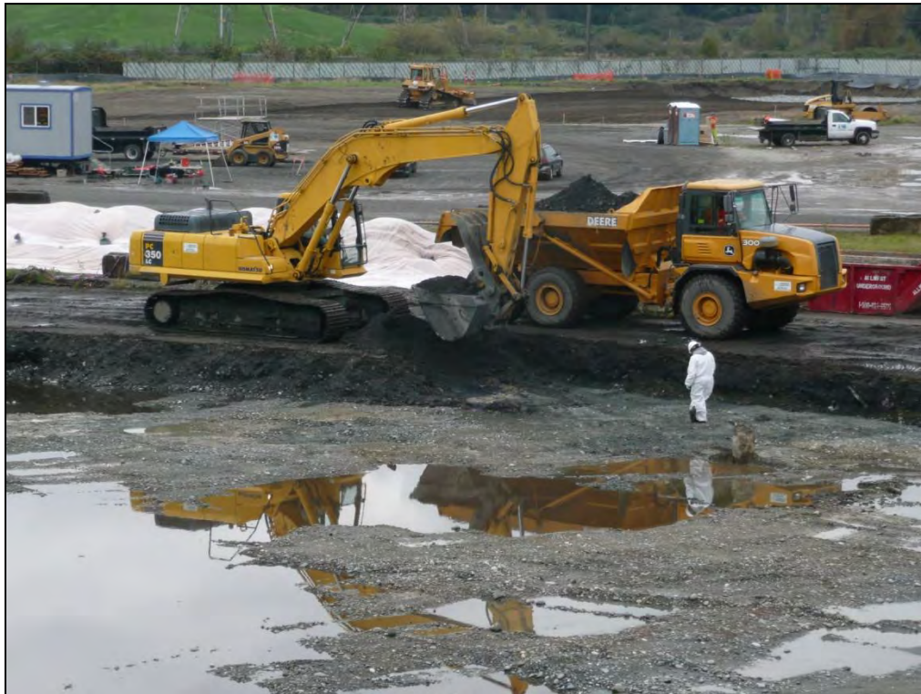
11. Looking southeast across the southern portion of the SPL Area during removal of SPL material.
