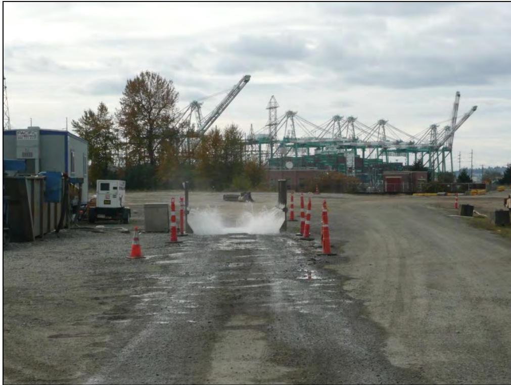
5. Looking southwest toward the automated wheel wash facility located adjacent to the site access road.
