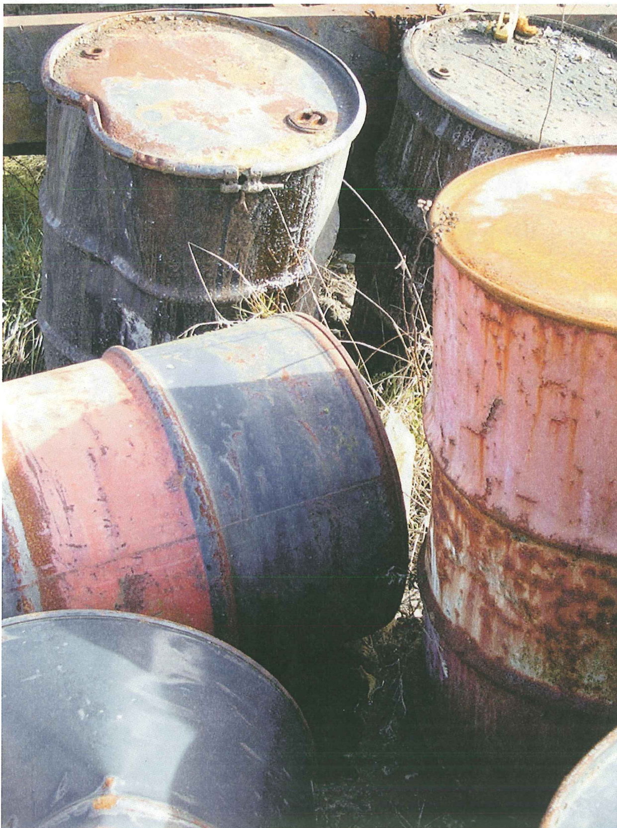
Treoil8: More bulging and leaking drums in the “200 Drum Area” shown in Treoil6a and 7. View is to the northeast.
