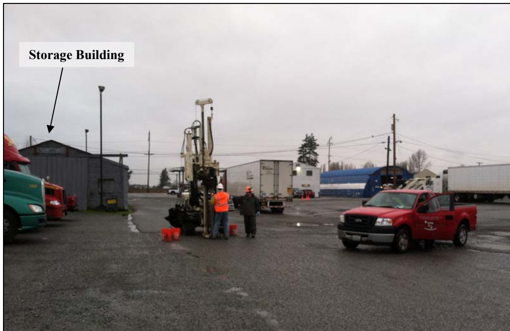
Photo 2. Borehole B-2 in progress. Storage to left, truck parking to right. Looking West.
