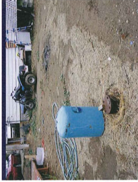
Photo 36 Wellhead at BK02.
