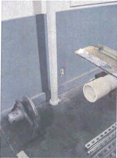
8-3-07 VIMS-5A Puget Sound Pipe (Facing South-East) – VIMS-5A Piping connecting to sump location
