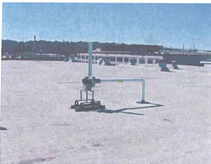
7-31-07 Exhaust fan unit - Mounted on roof of Hudson Bay Warehouse (Facing North-West)
