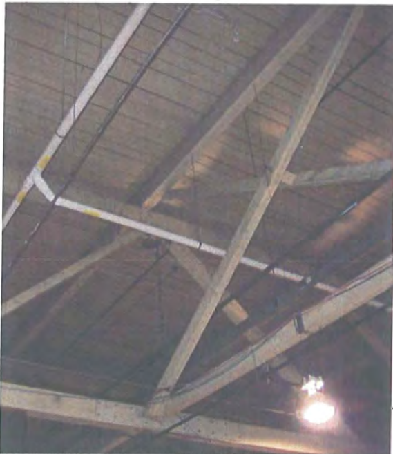
8-6-07 VIMS-4 Hudson Bay Warehouse (Facing West and up) – Piping connecting VIMS-3 and VIMS-4
