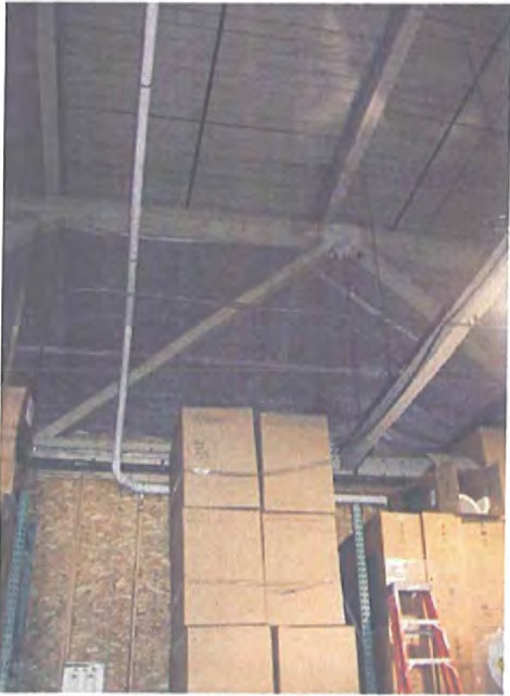
8-2-07 VIMS-3 Hudson Bay Warehouse (Facing West) - Piping from exhaust fan to VIMS-3
