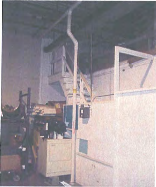
8-6-07 VIMS-5B Hudson Bay Warehouse (Facing North East) – Piping installed to the sump at VIMS-5B.
