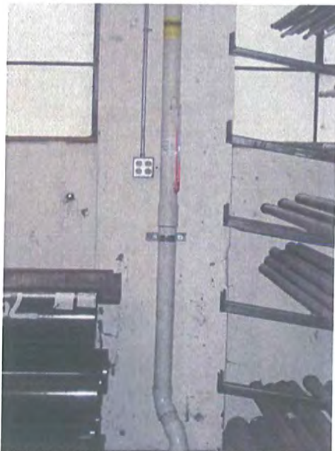
8-7-07 VIMS-1 -Puget Sound Pipe (Facing North) - shows manometer and signs attached indicating contacts regarding the system
