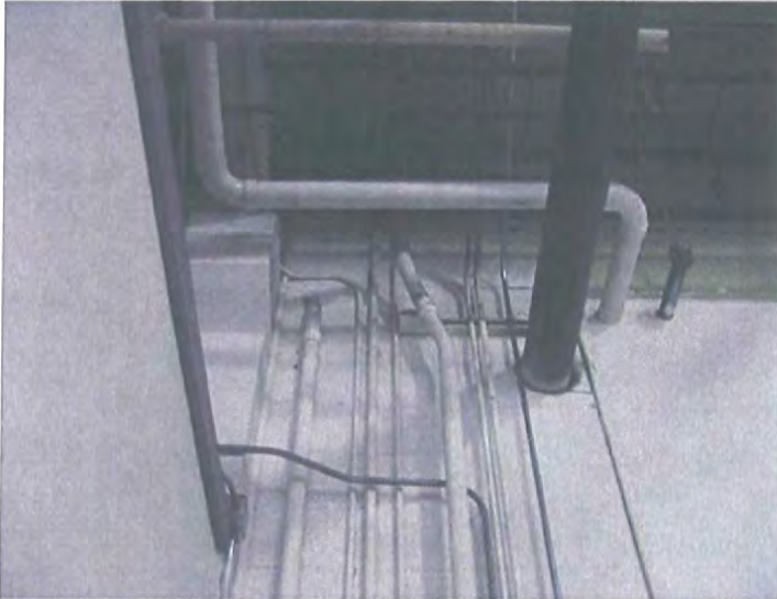
8-3-07 VIMS-5A Puget Sound Pipe (Facing South and Up) – Piping coming through Hudson Bay internal wall to Puget Sound Pipe.
