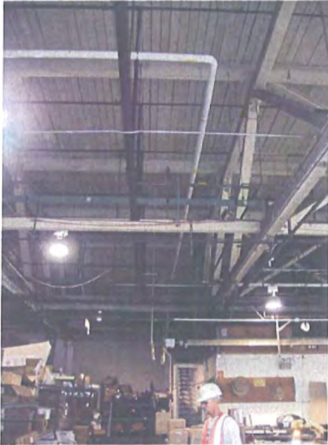
8-6-07 VIMS-4 Hudson Bay Warehouse (Facing North) – Piping network from exhaust fan to VIMS-5B
