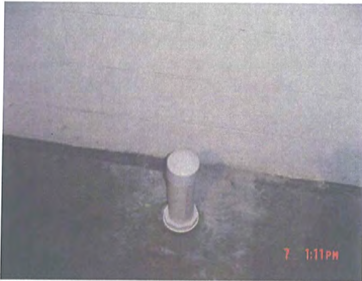
6-7-07 VIMS-4 Hudson Bay Warehouse (Facing North) – Capped Riser after excavation of sump
