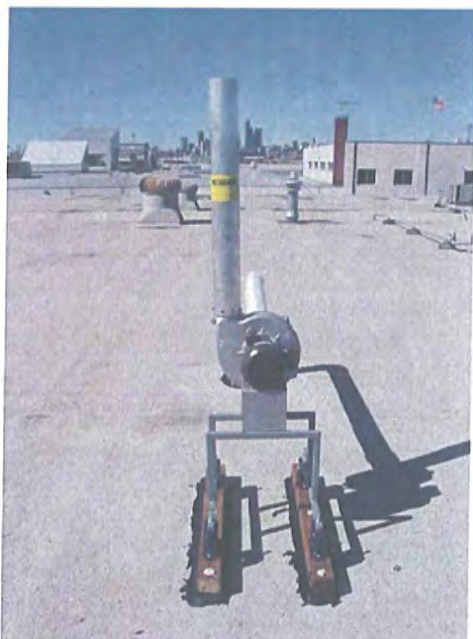
7-31-07 Exhaust fan unit - Mounted on roof of Hudson Bay Warehouse (Facing North)
