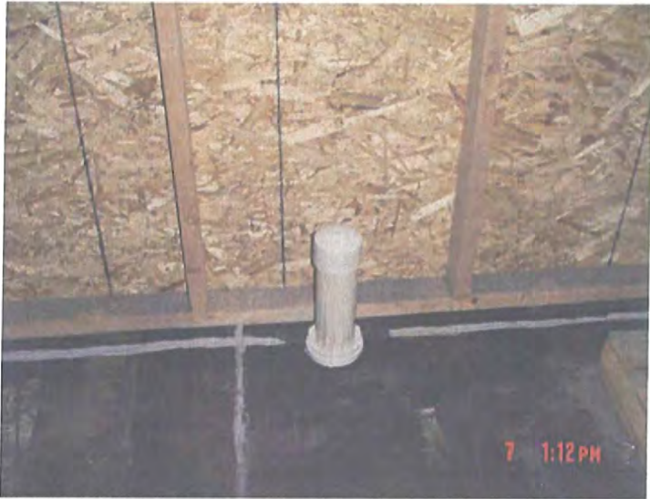
6-6-07 VIMS-3 Hudson Bay Warehouse (Facing West) – Capped Riser after excavation of sump
