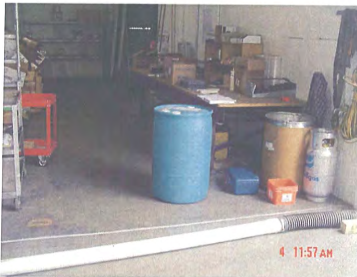
6-4-07 VIMS-1 Puget Sound Pipe Warehouse (Facing North) – Shows polyurethane sealing and installation vent piping from vacuum blower.
