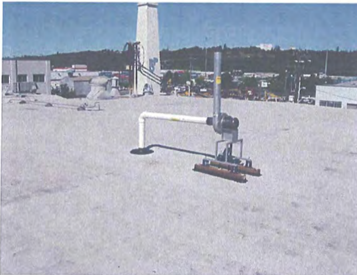
7-31-07 Exhaust fan unit - Mounted on roof of Hudson Bay Warehouse (Facing North-East)
