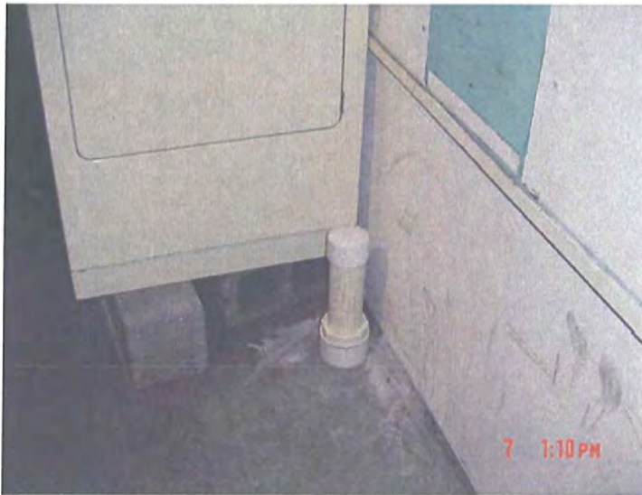
6-7-07 VIMS-5B Hudson Bay Warehouse (Facing Northeast) – Capped Riser after excavation of sump
