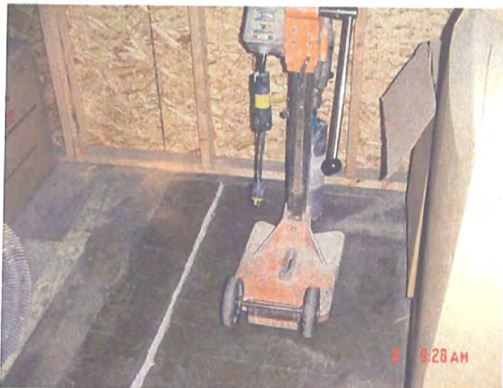
6-6-07 VIMS-3 Hudson Bay Warehouse (Facing West) - Drill set up to core out concrete
