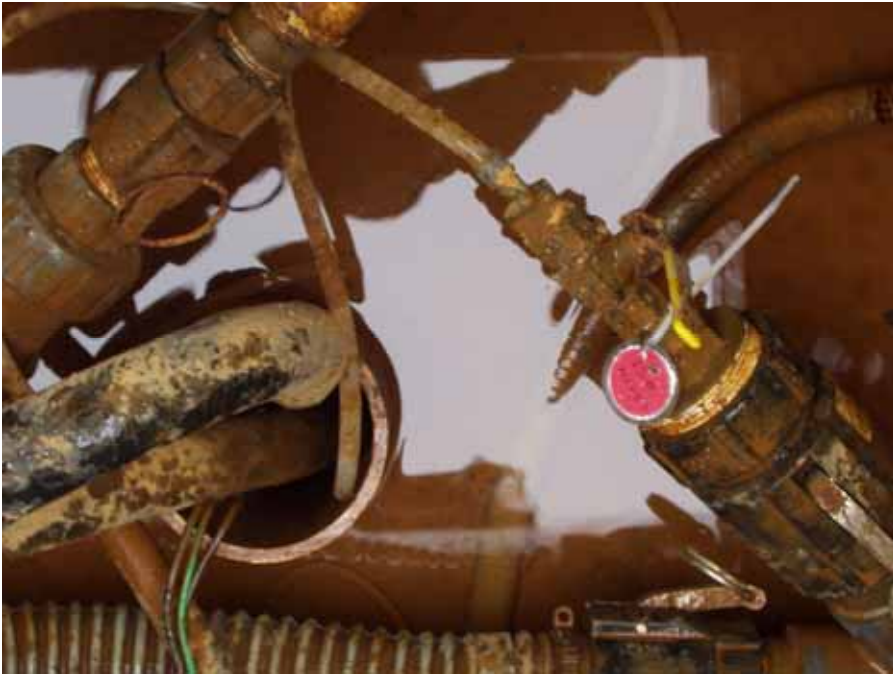
Recovery well RW-1 and sample port A4487 (shown with a red sample identification tag).
