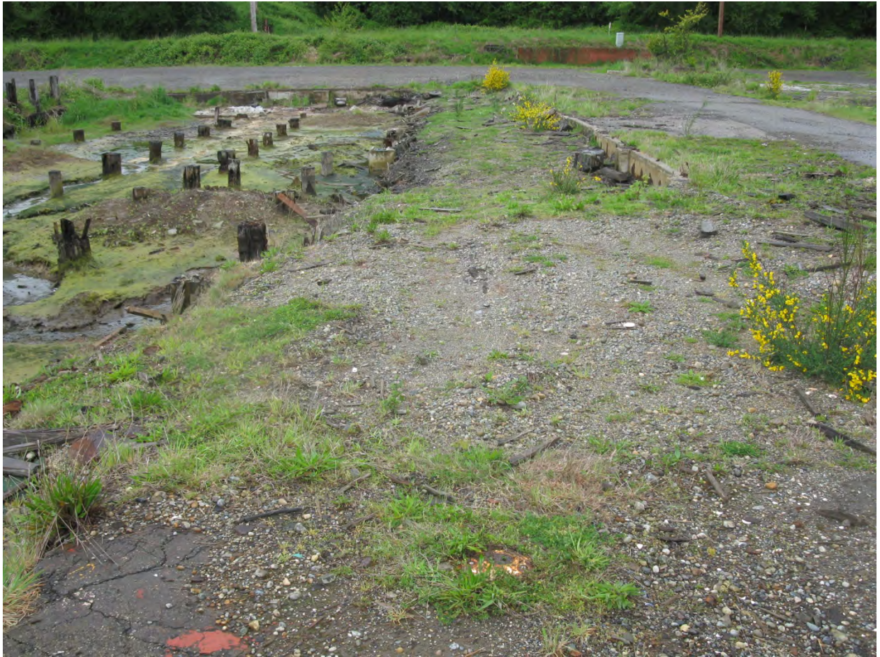
Photo 2: View of pilings and the concrete foundation on the north side of the former Maintenance Building. Well MW-6 (to be decommissioned) is in the foreground.
