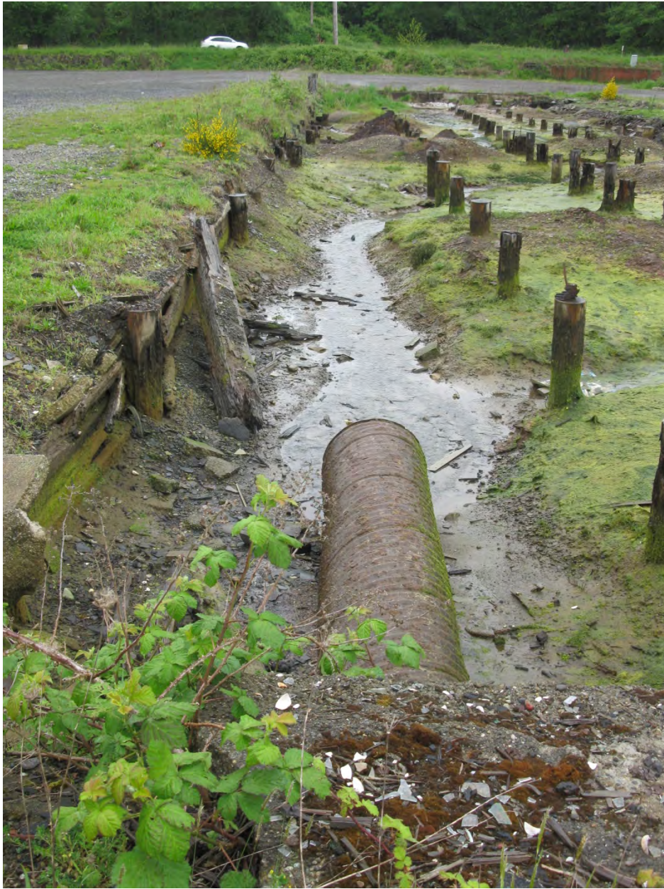
Photo 5 : View looking west toward West Bay Drive above the 30-inch diameter stormwater pipe at the east end of the former Maintenance Building.
