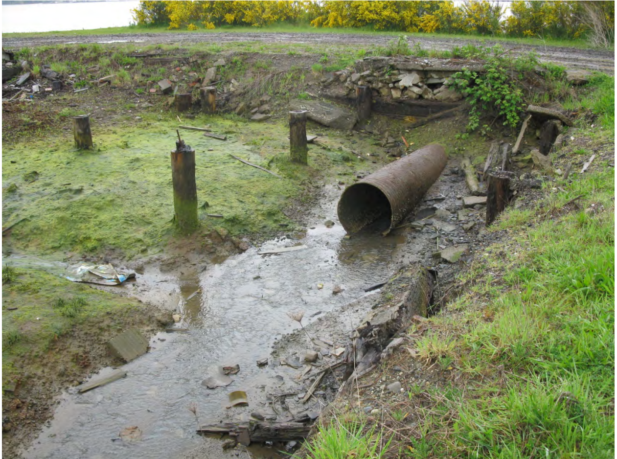
Photo 1 : View of upstream end of 30-inch diameter stormwater pipe.
