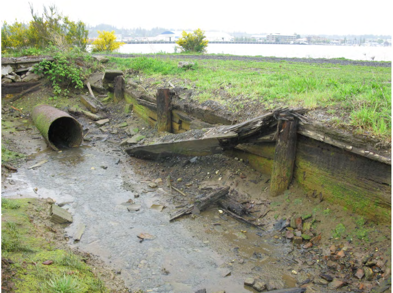
Photo 4 : View of wooden timber retaining wall near the southeast corner of the former Maintenance Building.
