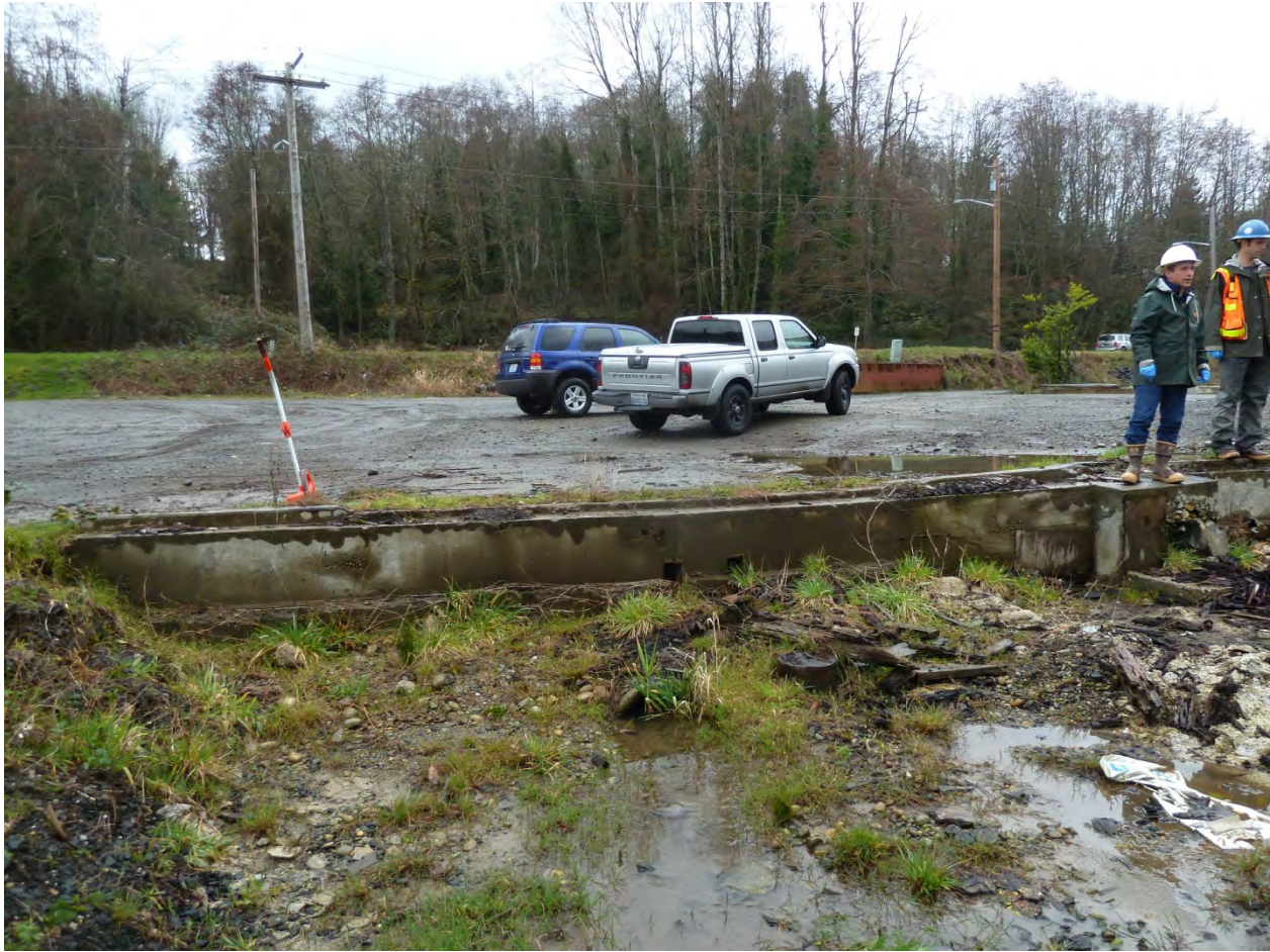
Photo 3 : View of concrete foundation at the west end of the former Maintenance Building. Note that this foundation contains and/or overlies a 15-inch diameter stormwater pipe which is to remain in-place. (Photo courtesy of GeoEngineers).
