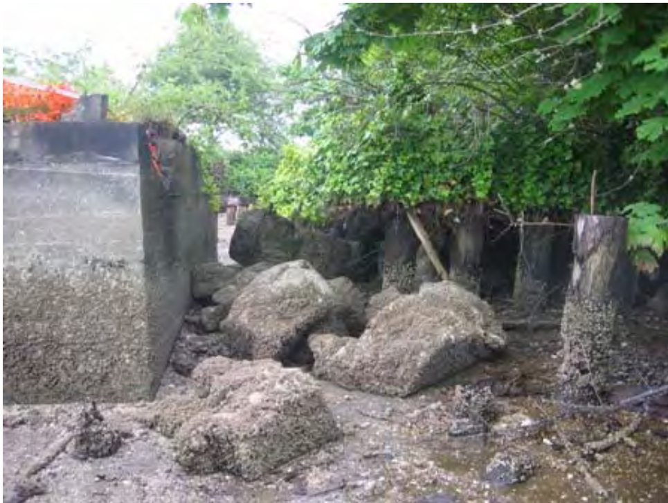
Photo 8 Beach substrate, concrete debris, and derelict piling, looking south
