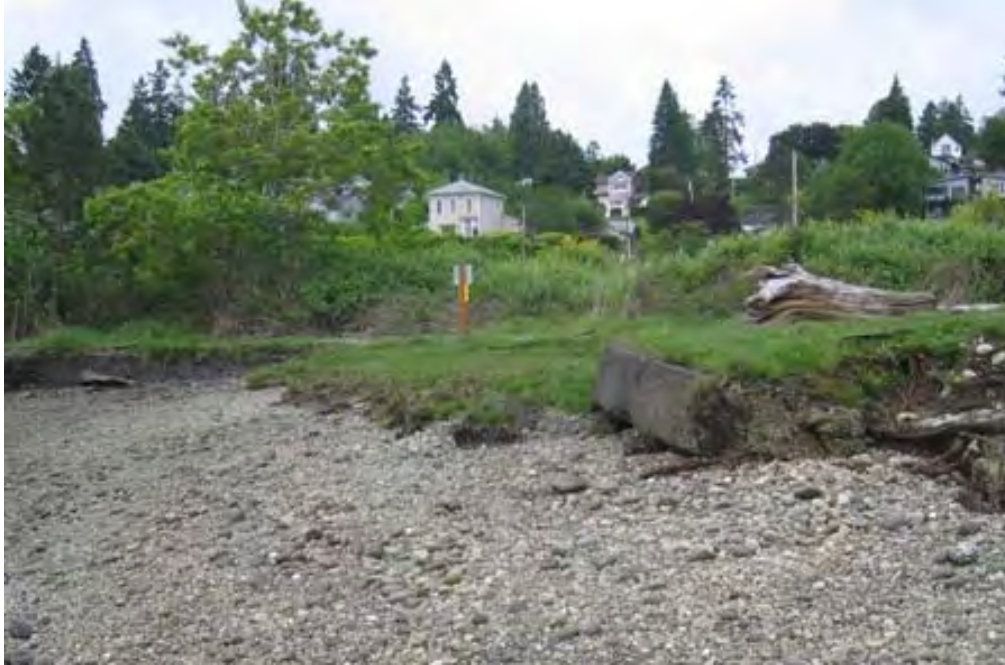
Photo 10 Erosion at the park shoreline, looking southwest
