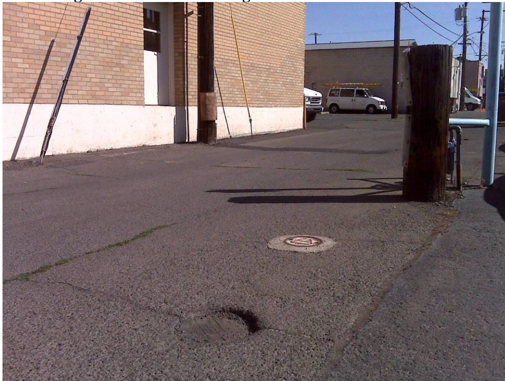
Photo 4: Monitoring Wells South of Building – from the southwest
