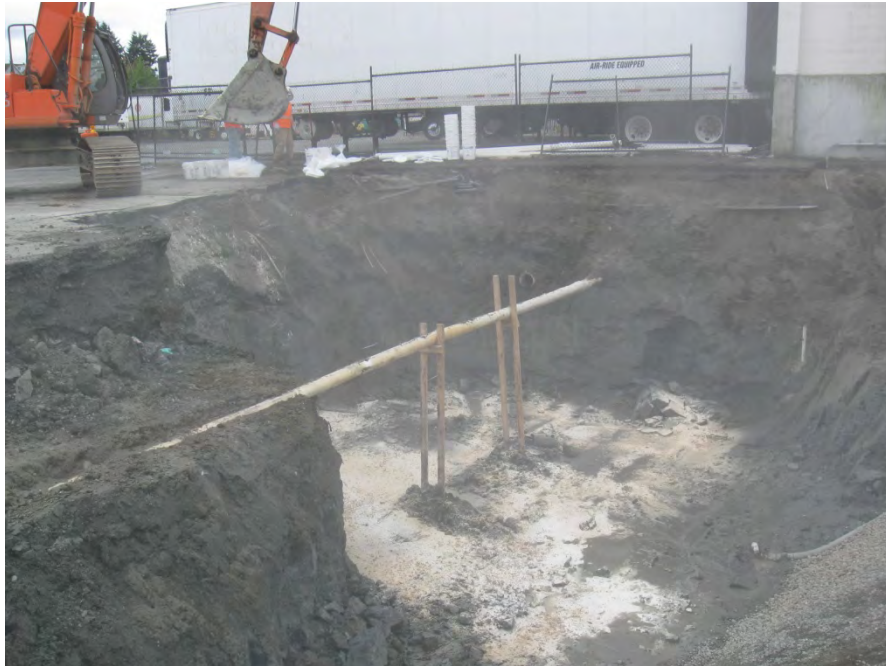
Photo 7: Sanitary Sewer Line Protected during Construction (Note Regenesis Products Spread on Excavation Bottom), 7/26/2011
