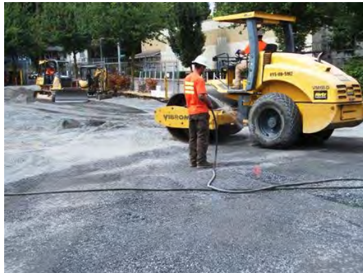
Water Being Added to 5/8" Crushed Minus While Compacting With Smooth Roller Drum
