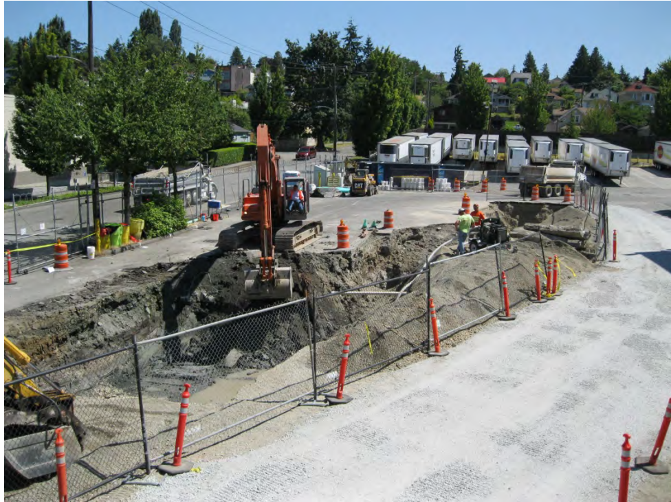
Photo 9: Excavation in Northwest Corner (Note Temporary Truck Lane Over Backfilled Southern Portion of Excavation), 7/30/2011
