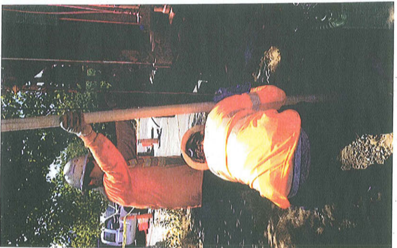
Figure 18. Cascade Drilling, LP is installing white PVC well casing for new groundwater compliance well located a public right-of-way at N Northlake Place at Metro Lake Union Site.
