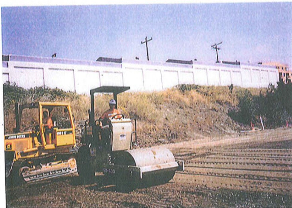
Figure 4. Former AST tank farm area with all tanks removed and shallow soils with sand blast grit and paint chips removed that had shown elevated metal concentrations. This was Metro/Chevron Cleanup Action Plan phase 1 completed in October 1999-January 2000.
