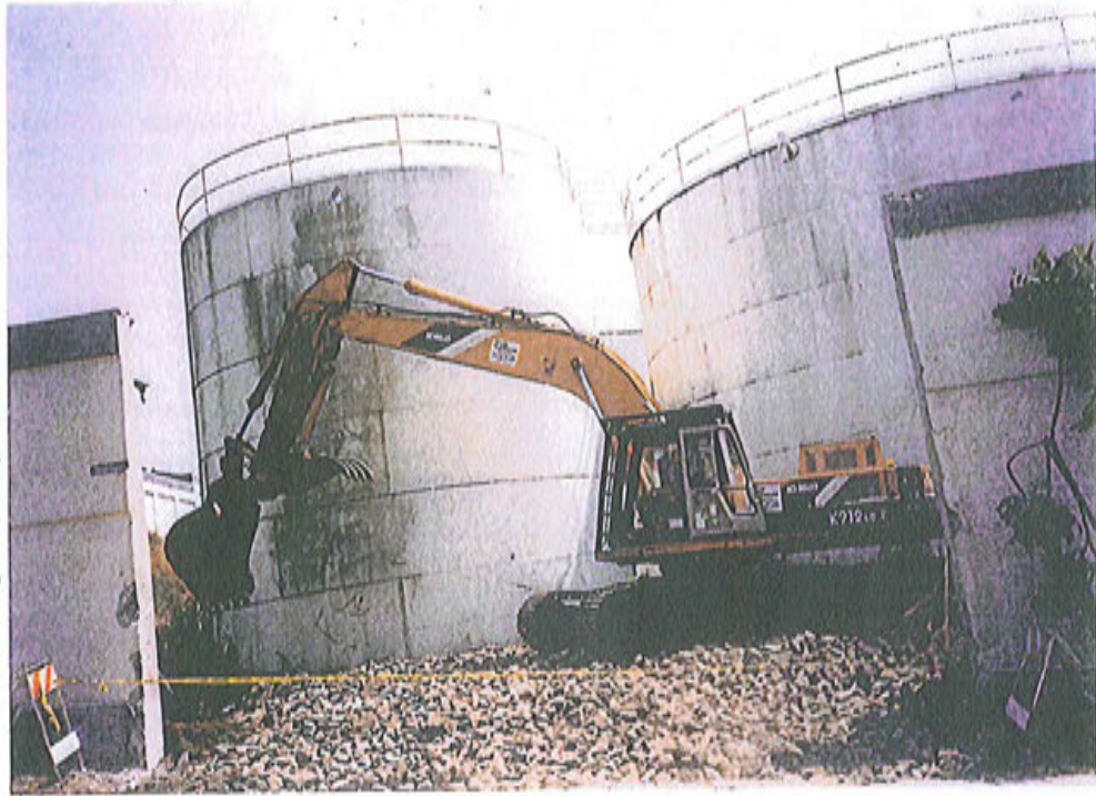
Figure 3. Metro Lake Union Site former Chevron Bulk Terminal #100-1327 above ground petroleum storage tank (AST) farm located at North Yard to begin demolition with excavator to cut and dismantle ASTs for metal recycling in October 1999.
