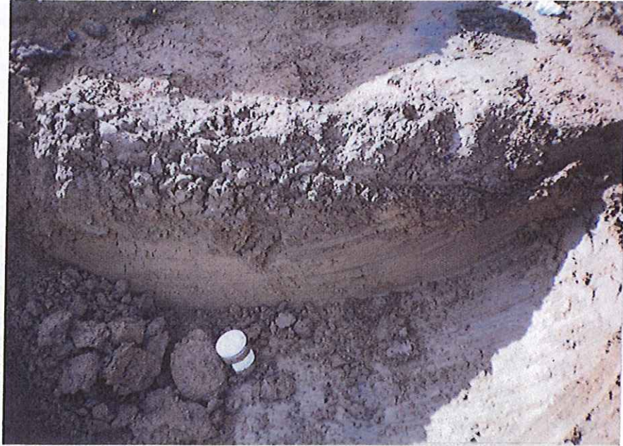
Photo 9 - Overhead view of west end of former fuel island excavated to 2' BGS. Note sample jar (#15) at collection point, where soil around sample is clean (02/26/96).
