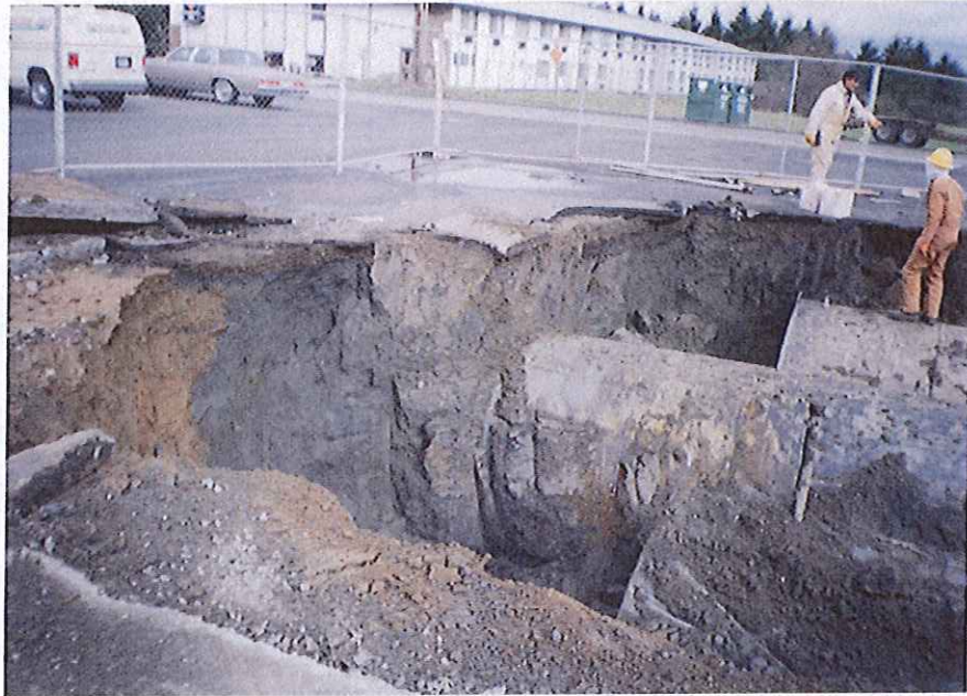
Photo 3 - Gray petroleum stained soil on south wall prior to excavation of tanks T1, T2, and T3 (02/23/96).
