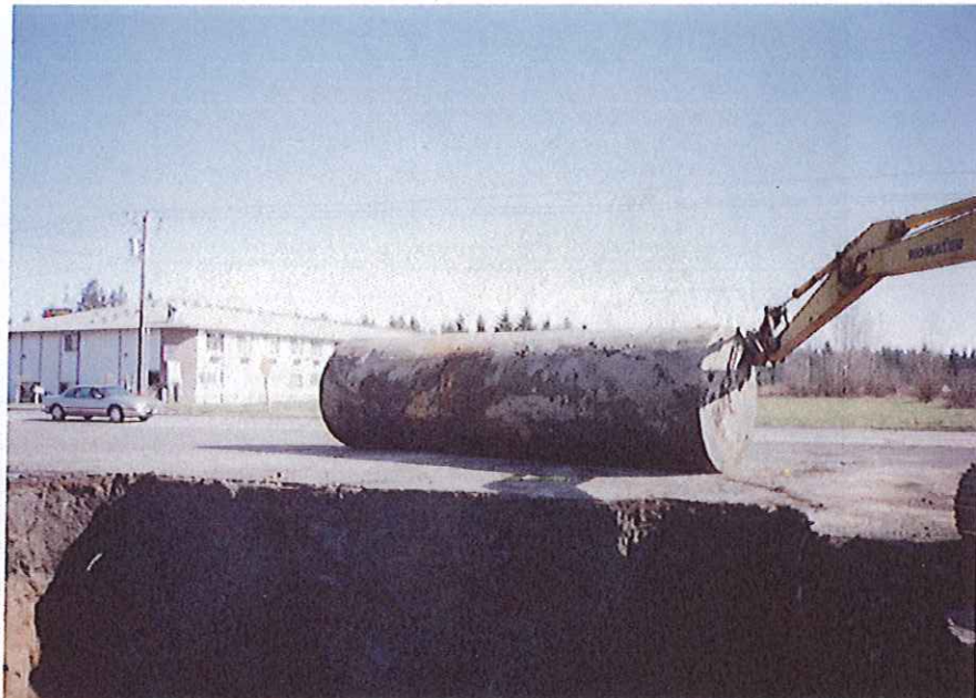
Photo 8 - View of tank T2 after excavation. Tank appeared to be in good condition with only minor surface rust (02/26/96).
