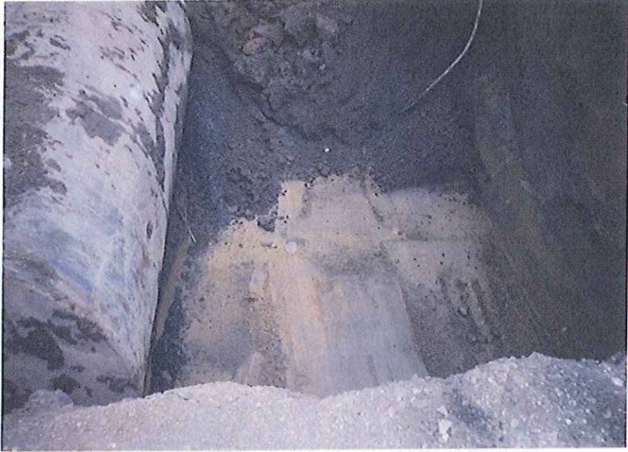
Photo 5 - Brown colored native soil in floor of excavation at 12' BGS is "clean" per laboratory test results (02/23/96).
