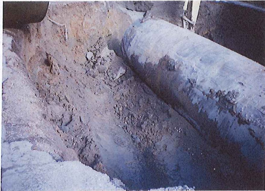
Photo 7 - Gray stained soil on floor of tank pit after removal of tank T3. Tank T2 is on right in photo (02/26/96).
