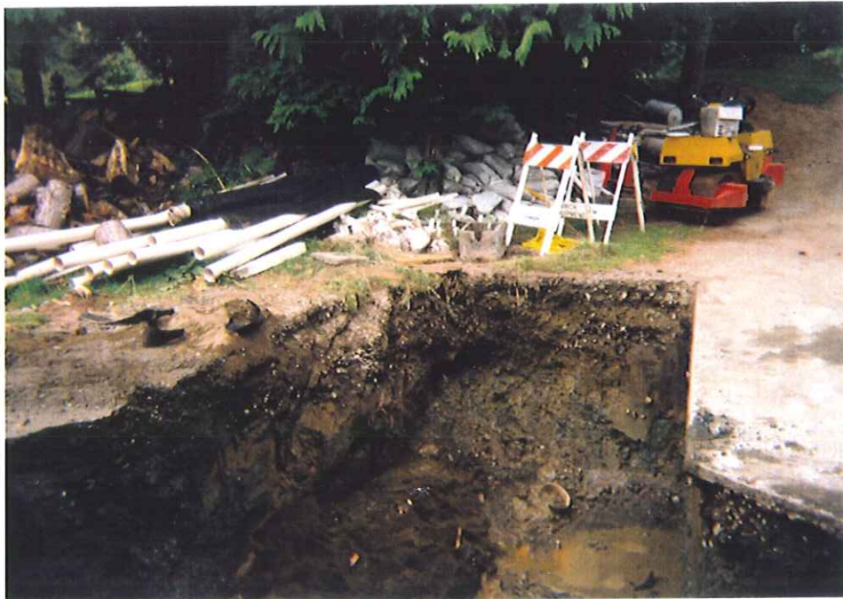
PIT FROM TANK #2 AT MAINTENANCE BUILDING
