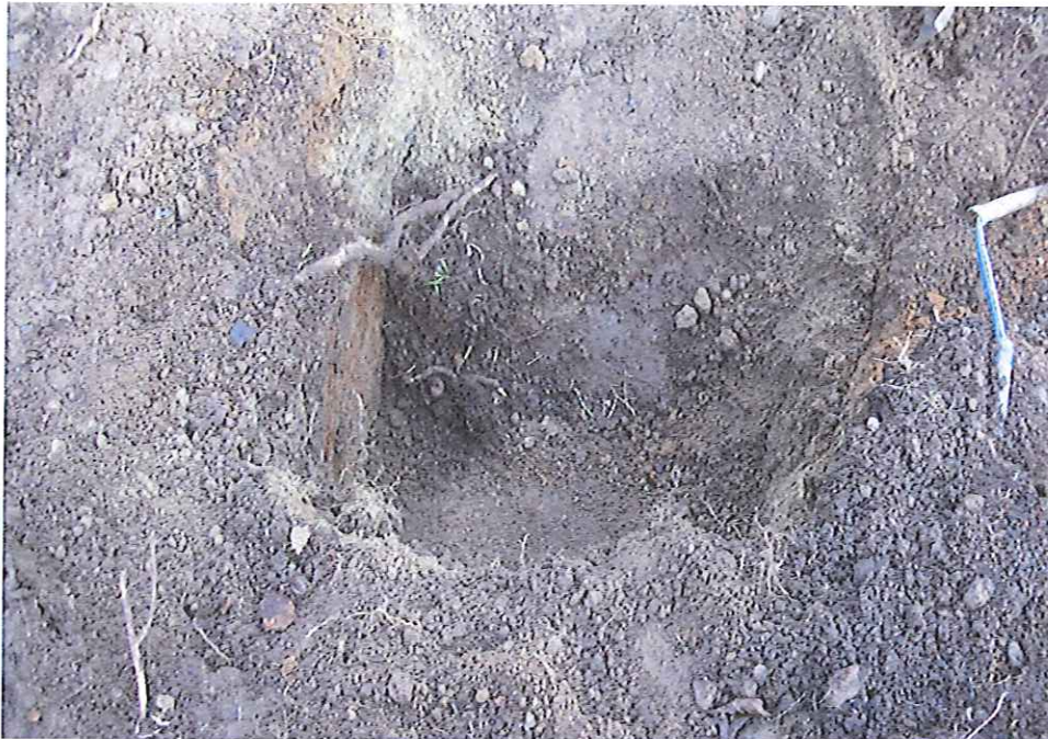
Looking south at the starter tank pit bottom subsequent to removal. No visual or olfactory indications of PCS noted.
