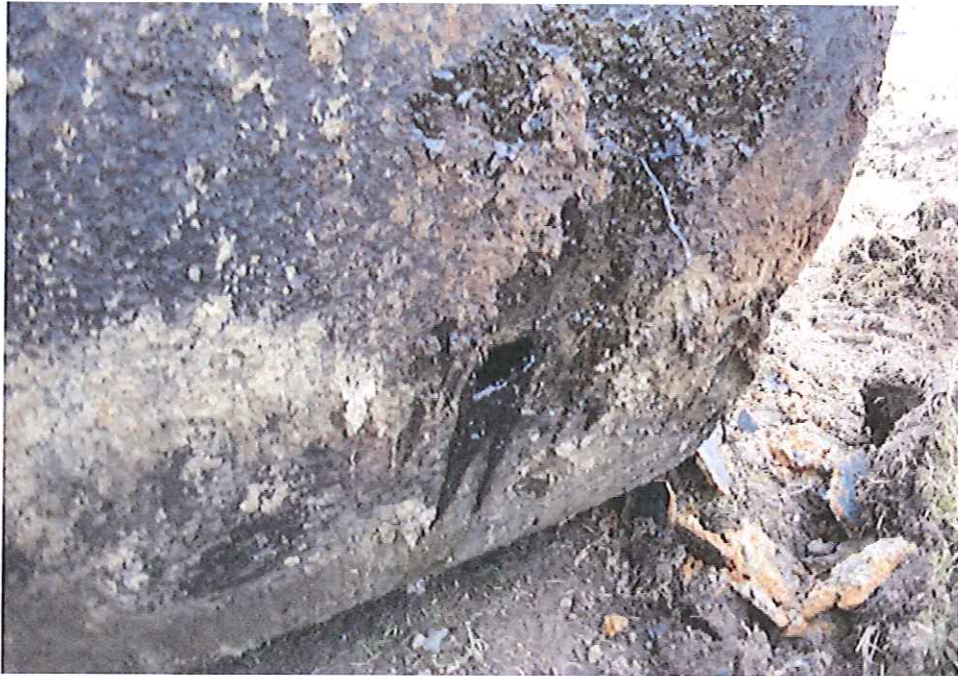
A large hole was discovered in the UST bottom. The tank had originally contained PS 300 (black oil) prior to being converted to a diesel heating fuel storage tank.
