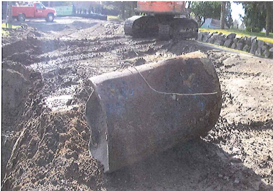
Removed 500 gallon gym site tank. No visual or olfactory indications of PCS noted.
