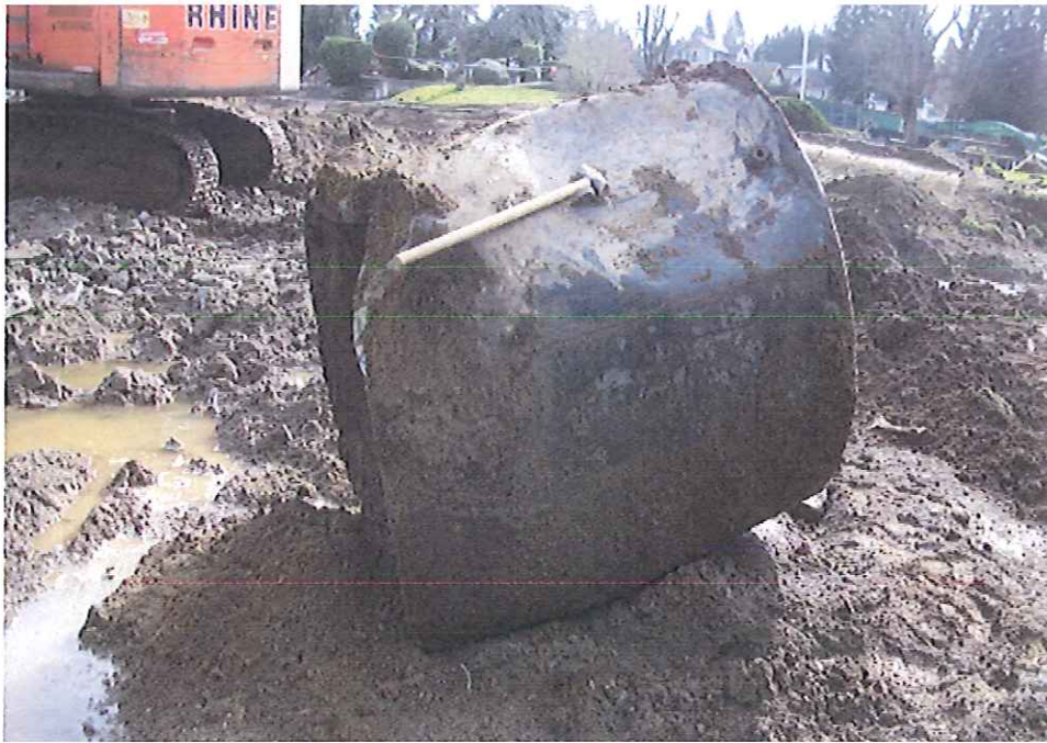
Removed Heather building tank was sized at 64" x 72" with a nominal capacity of 1,000 gallons.
