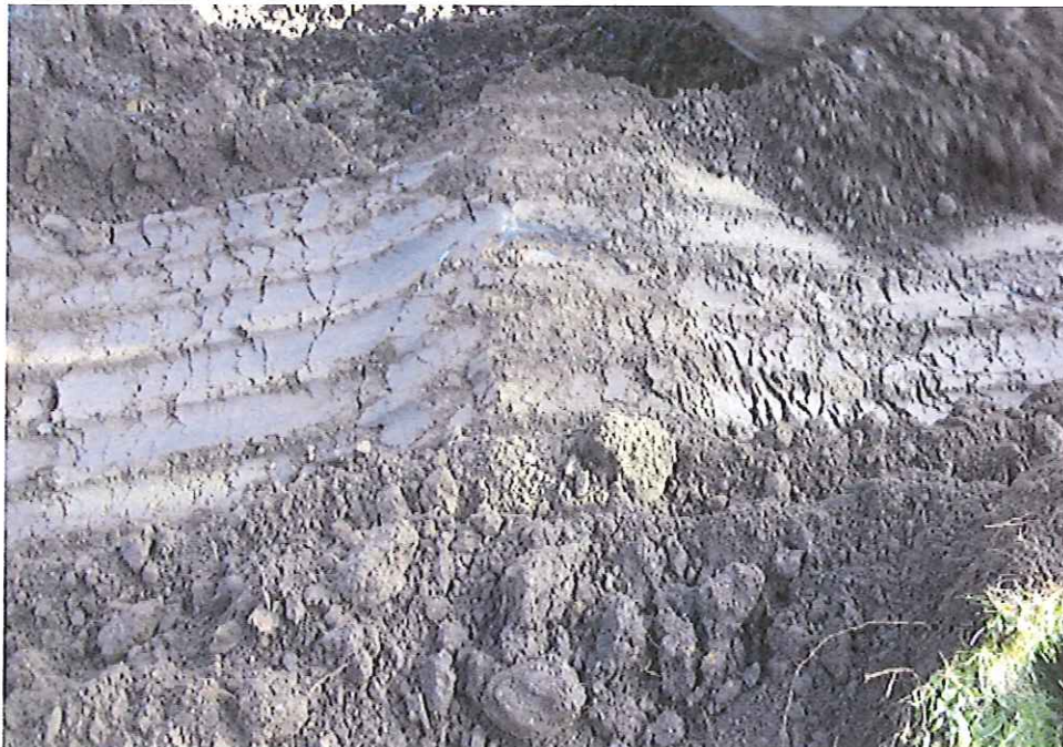
Heather building UST exposed under 12" of earth cover.
