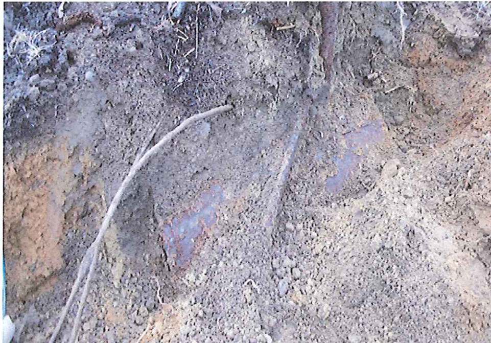
The additional diesel fuel starter tank discovered at the Holly building was exposed under 20" of earth cover.
