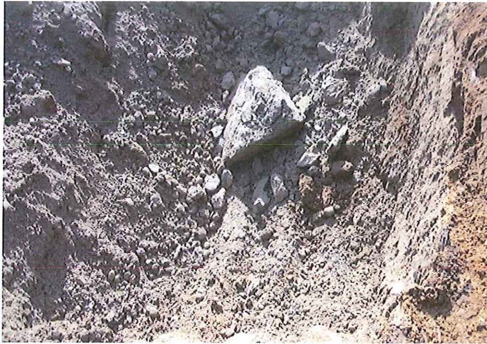
Gym UST tank pit bottom. Soil sample analytical results were at the non-detect level.
