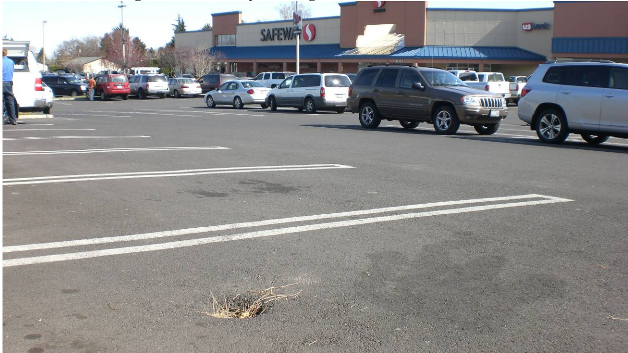
Photo 1: Monitoring Well in Safeway Parking Lot w/ No Lid – from the northwest
