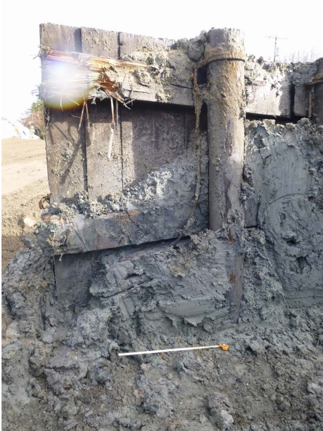
Figure 5: Same section of bulkhead as Figure 4, closer view (tape at 2 feet and view to east).
