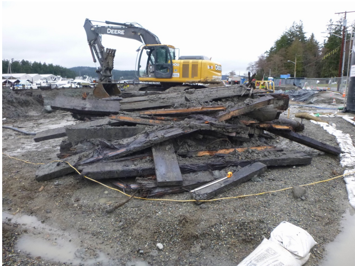
Figure 6: Overview of removed portions of the bulkhead, showing variable lengths and widths of creosote-treated components to the bulkhead (view to north).
