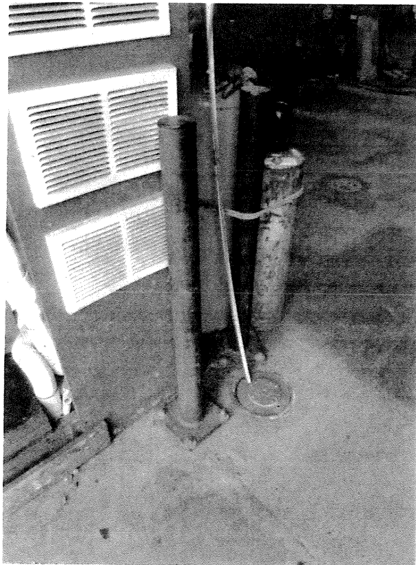
FEED LINE FROM SUBMERSIBLE PUMP IN WELL #2
